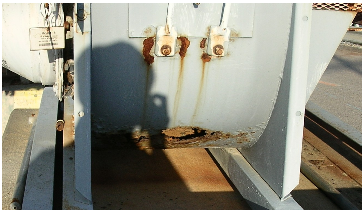
Figure 7. Breach of annulus fan housing due to accumulation of water.
