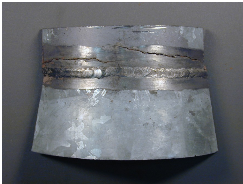
Figure 6. Section of ventilation ductwork removed from the exhaust of the purge ventilation system. Two cracks are evident. A third crack, located on the opposite side of the weld, occurred on the inside surface but did not penetrate to the exterior. Magnification is 1.25 X.
