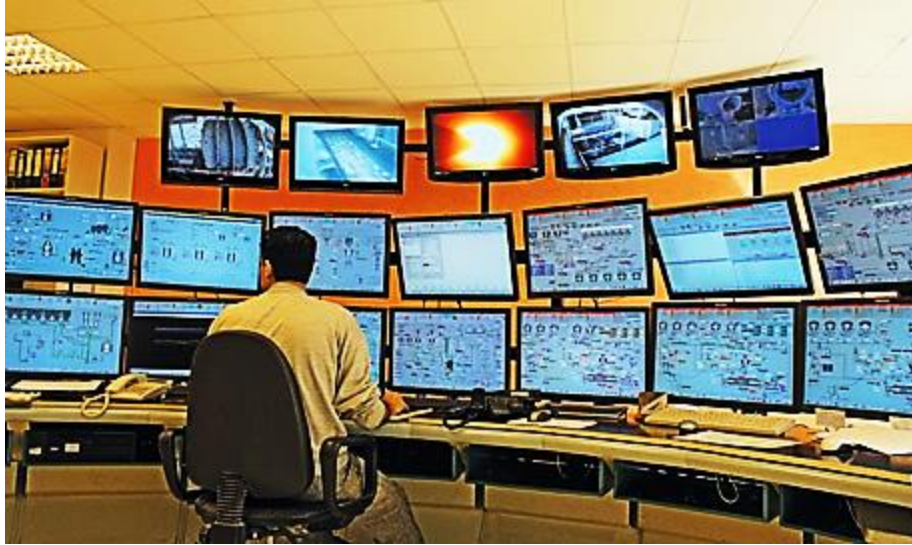
Fig 1.18: A typical DCS CCR and graphical interface operates plants easily (taken from [24])
