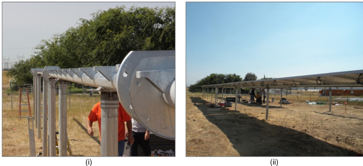
Figure 33: Views during alpha installation of T0 v2 tracker. (i) New torque tube design featuring factory-welding PV mounting saddles and bolted connections between segments. (ii) Alpha system with PV modules installed, demonstrating alignment achieved with new design.
