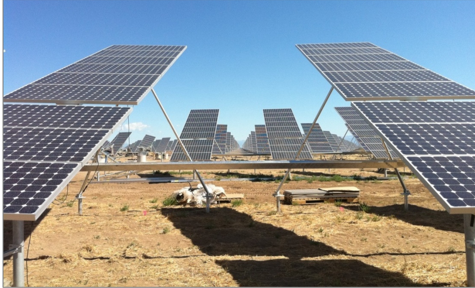
Figure 31: T20 v2.3 & 128-cell module installation underway at 24-MWp array in Alamosa, CO
