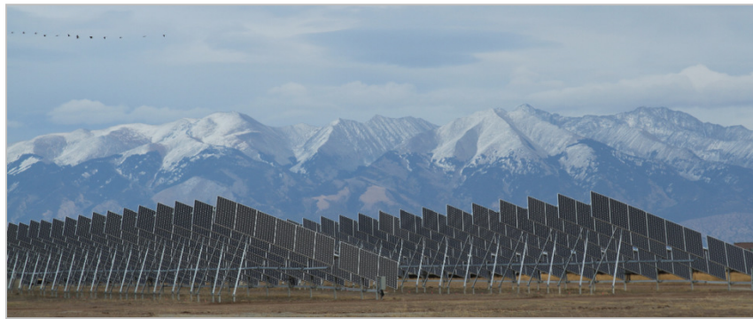
Figure 32: T20 v2.3 trackers following commissioning
