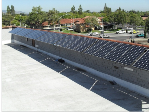
Figure 77: Two strings of SunPower modules installed in Los Gatos for SAI inverter reliability study
