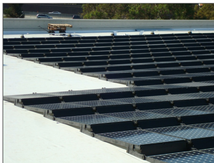
Figure 23 Portion of 1-MW T5 installation in Santa Clara, California
