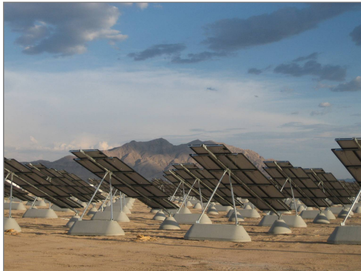
Figure 28: 14-MWp T20 v1 tracker system deployed at Nellis Air Force Base
