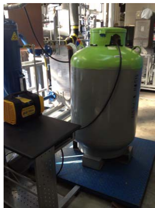
Figure 40. Tank of the new working fluid
