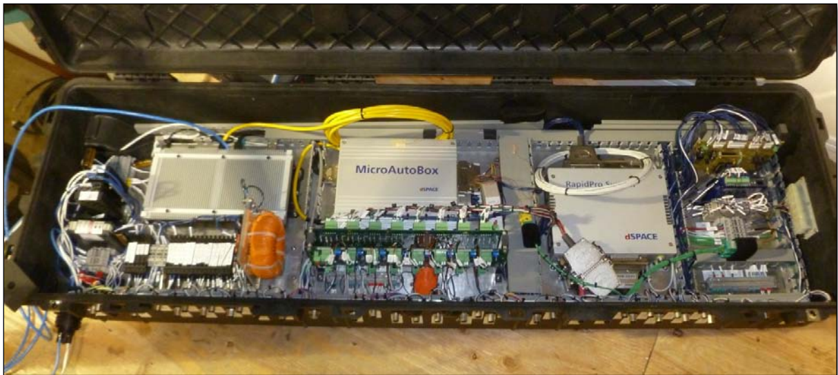
Figure 5 - SeaRay's SCADA and control hardware in a watertight enclosure.
