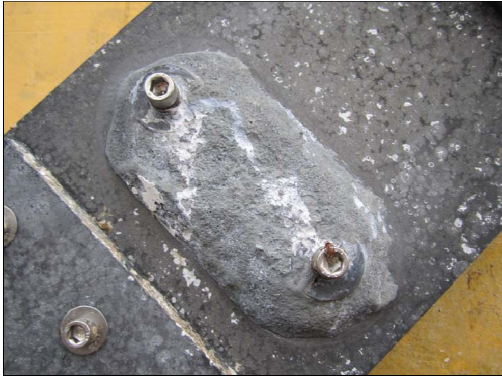
Figure 45 - Degraded zinc anode after deployment.
