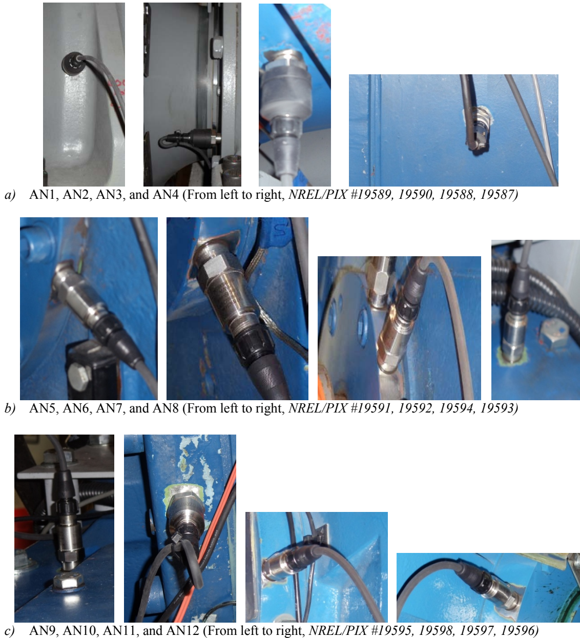
Figure 2.8. Physical sensor installation
