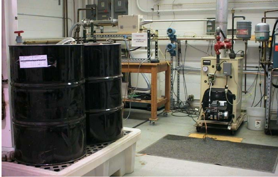
Figure 4. Cast iron boiler fueled with ULS diesel fuel
