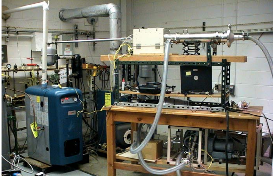
Figure 7. Gas-fired condensing boiler
