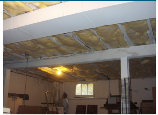
Basement ceiling insulation. When this home was remodeled for energy efficiency, the basement ceiling was extensively air sealed and then insulated with unfaced batts (Photo Source: PNNL).
