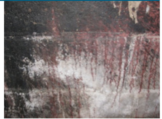
Wet masonry. Avoid insulation strategies that increase moisture retention in masonry walls. Wet masonry can develop mold and efflorescence, a chalky salt residue (Photo Source: PNNL).
