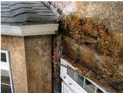
Improper flashing can allow rain water into walls, causing significant damage (Source: DryFlekt Products, Inc.).
