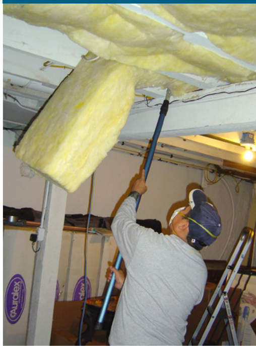
Basement ceiling insulation. Unfaced fiberglass batts are installed in the ceiling of this basement in Portland, Oregon (Photo Source: PNNL).
