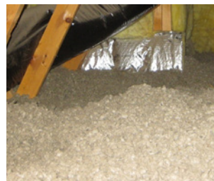
Loose fiberglass insulation
