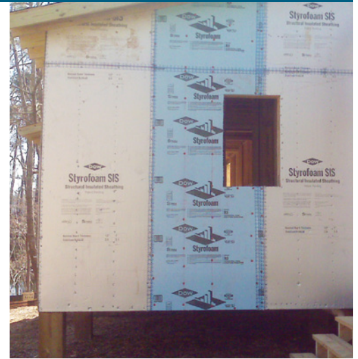
Exterior rigid foam. Rigid foam insulation is installed on the exterior of a new framed home in Georgia. The rigid foam takes the place of OSB wall sheathing (Photo Source: IBACOS).
