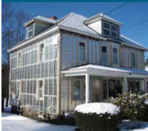
Exterior rigid insulation. A complete renovation of this Massachusetts home included insulating the walls with exterior rigid insulation and interior cellulose (Photo Source: BSC).
