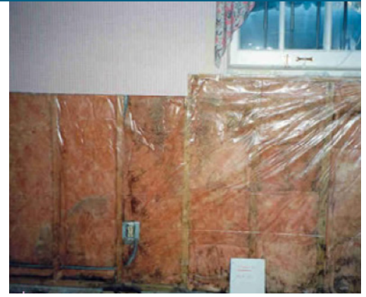
Vapor retarders and mold. Vapor barriers like this polyethylene sheet can trap moisture in walls. The damp fiber insulation in this wall developed mold and odors (Source: BSC).
