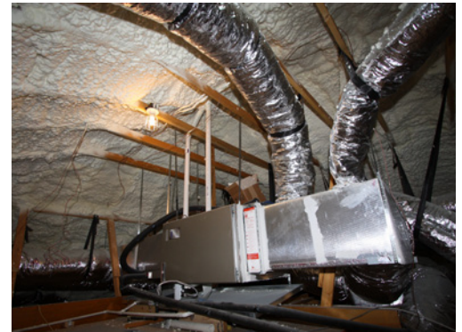
(Top) Spray foam insulation. Spray foam was used to simultaneously air seal and insulate this ventilated attic. Baffles installed in each rafter bay keep the insulation from blocking the soffit vents (Photo Source: WSU Energy Office).
