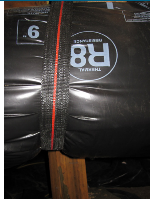
All ducts should be laid straight and adequately supported. Flex ducts should be stretched tightly; loose, sagging ducts can greatly restrict air flow (Photo Source: PNNL).
