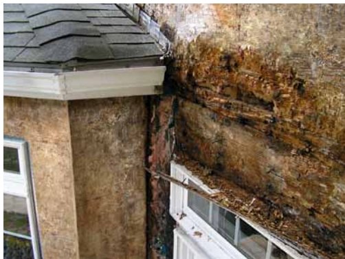
Improper flashing can allow rain water into walls, causing significant damage (Source: DryFlekt Products, Inc).
