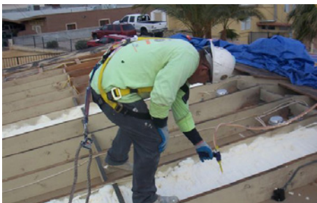
Closed-cell spray foam fills the rafter bays of the vented cathedral ceiling.
