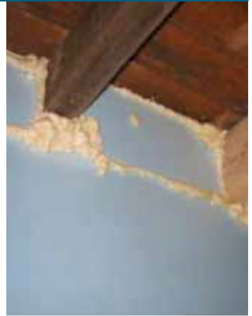
Interior rigid foam. To create an air barrier, seams of the rigid foam insulation were carefully sealed with spray foam (Photo Source: PNNL).
