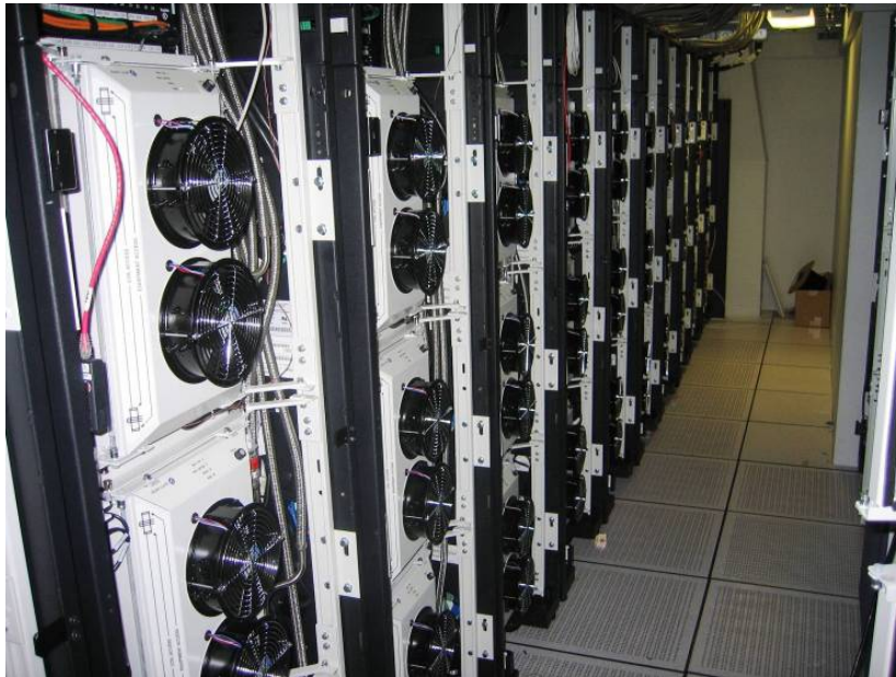
Figure 75: Alcatel-Lucent’s Modular Cooling Solution installed in ALU’s 17-rack, 100 kW Network Systems Integration and Test IPTV Laboratory in Plano, TX.
