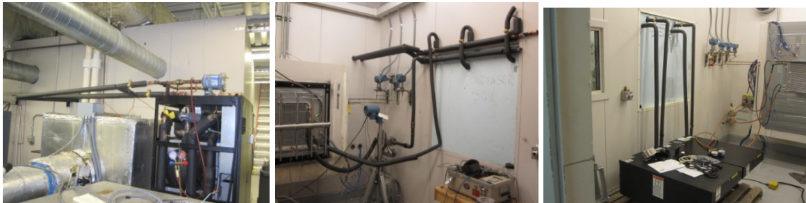
Figure 9: Pumping Station and air duct behind calorimeter room (a), test HX and manifold piping (b), and XDV modules (c).
