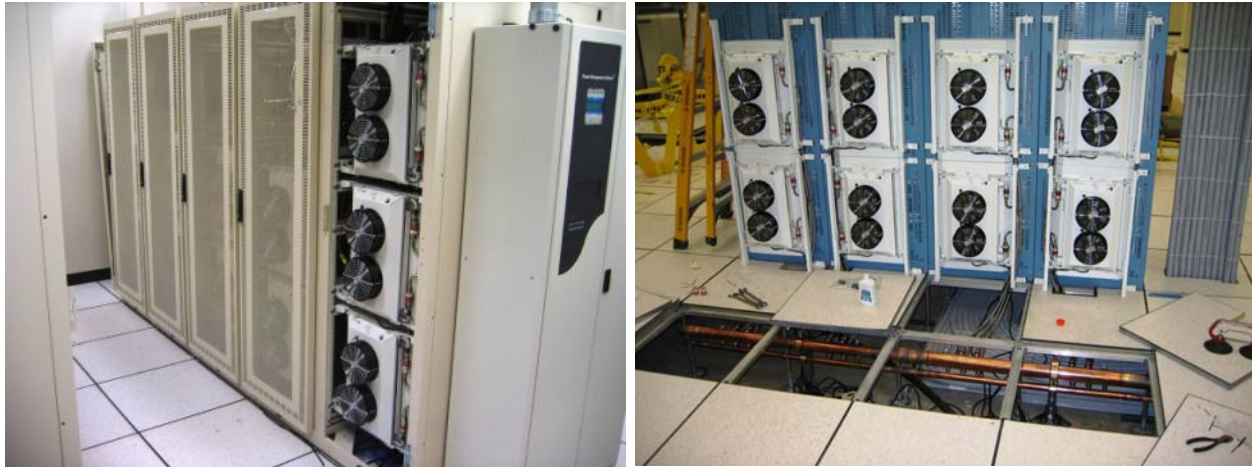
Figure 68: ALU facilities in Naperville, IL used for evaluation of layout of underfloor refrigerant piping: (left) Prototype Data Center; and (right) Adjacent Data Center. Note shelf-level modular cooling units attached to rectifier cabinets.
