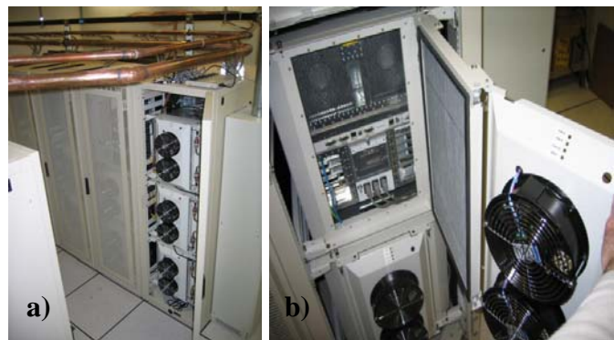
Figure 3: Photographs of 10-rack modular cooling system showing: a) overhead refrigerant piping and equipment racks outfitted with shelf-level heat exchanger / fan assemblies (left); and b) retractability of heat exchanger / fan assembly for equipment access (right).
