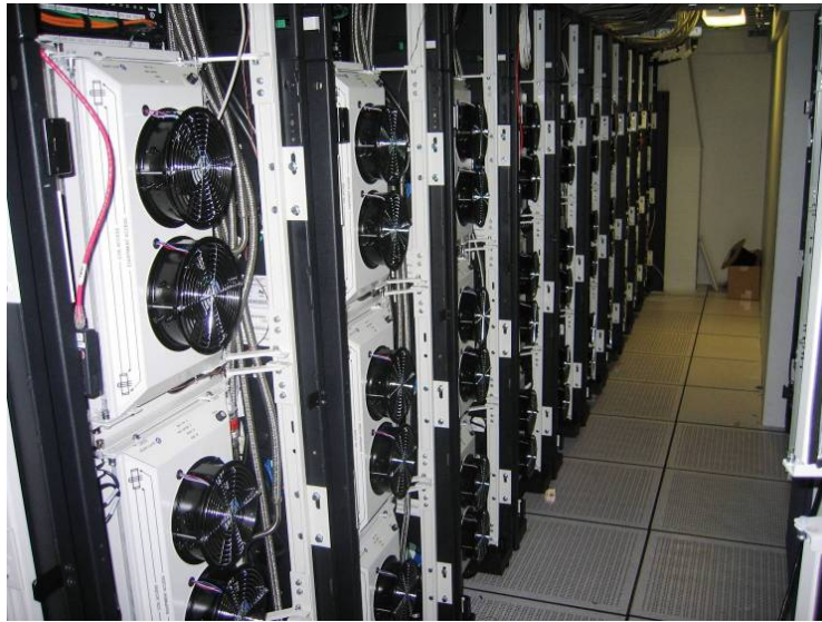
Figure 67: 17-rack 100 kW server farm (Server Farm 1) located in Plano, TX.
