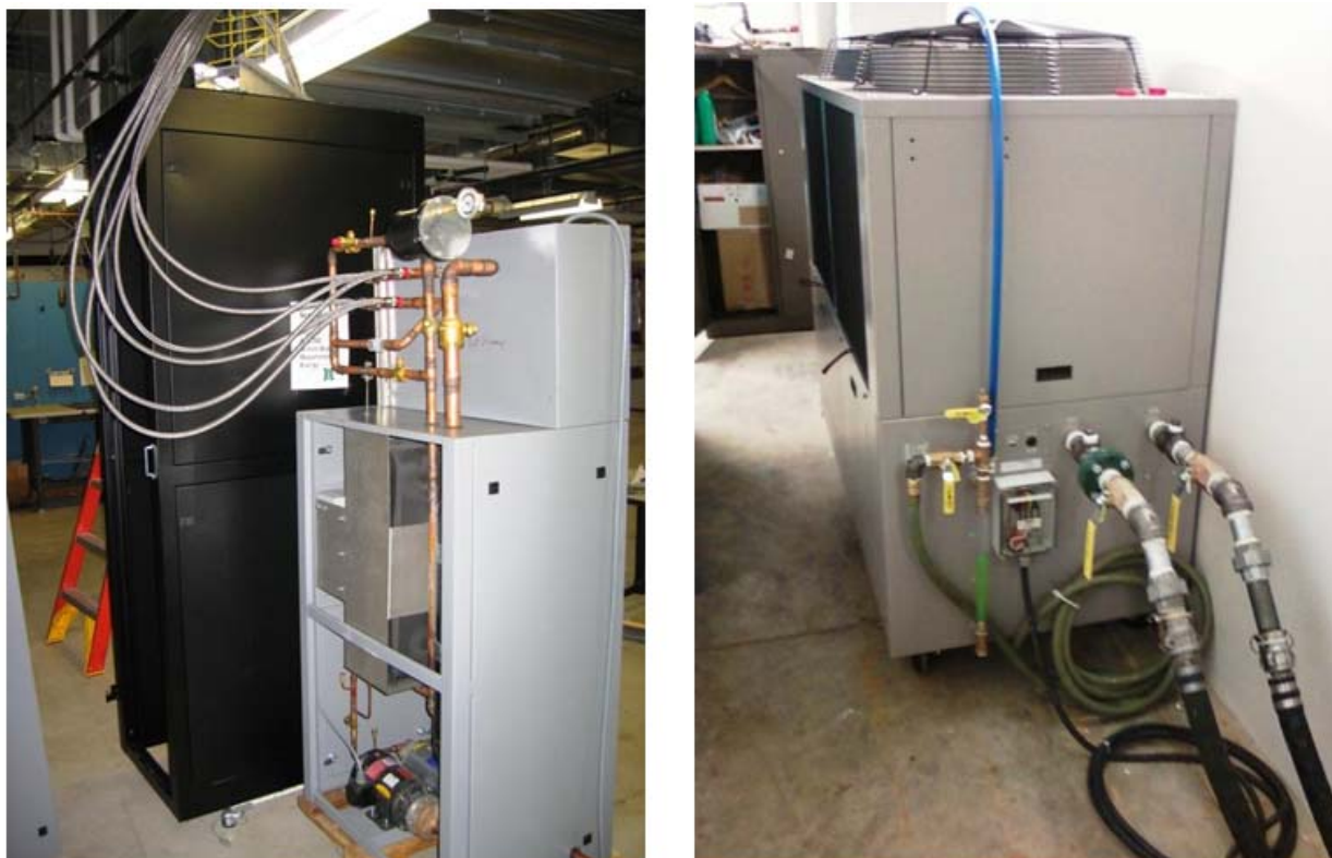
Figure 62: (left) chilled water pumping station (gray box) connected to 18 kW heat load (black box); and (right) portable chilled water plant.
