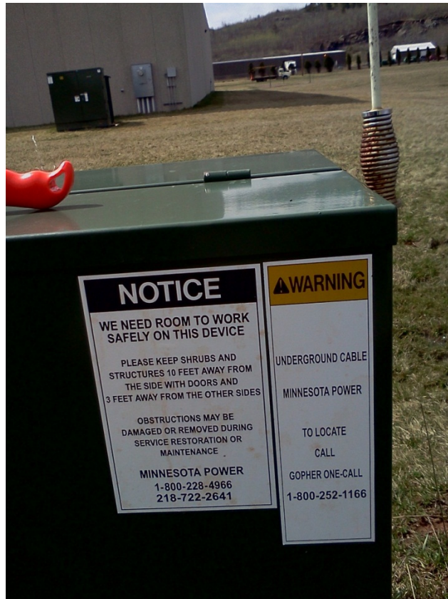
Figure 12. Potential electrical tie-in point for the PV system at the Atlas Industrial Park showing the IKONICS building and meter in the background
