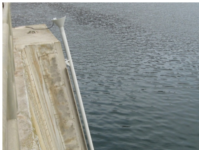
Figure 3.8. Trolley pipe mounted on a main pier of the John Day Dam powerhouse showing the cone used as a guide for trolley insertion.
