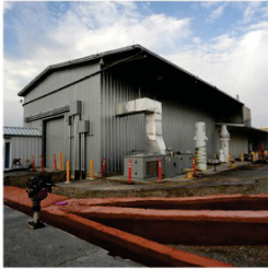
A portion of the new electrical distribution loop to provide double-ended feed for all facilities on the north side of MFC. The Experimental Fuels Facility (shown) is one of the R&D facilities benefitting from this power expansion.
