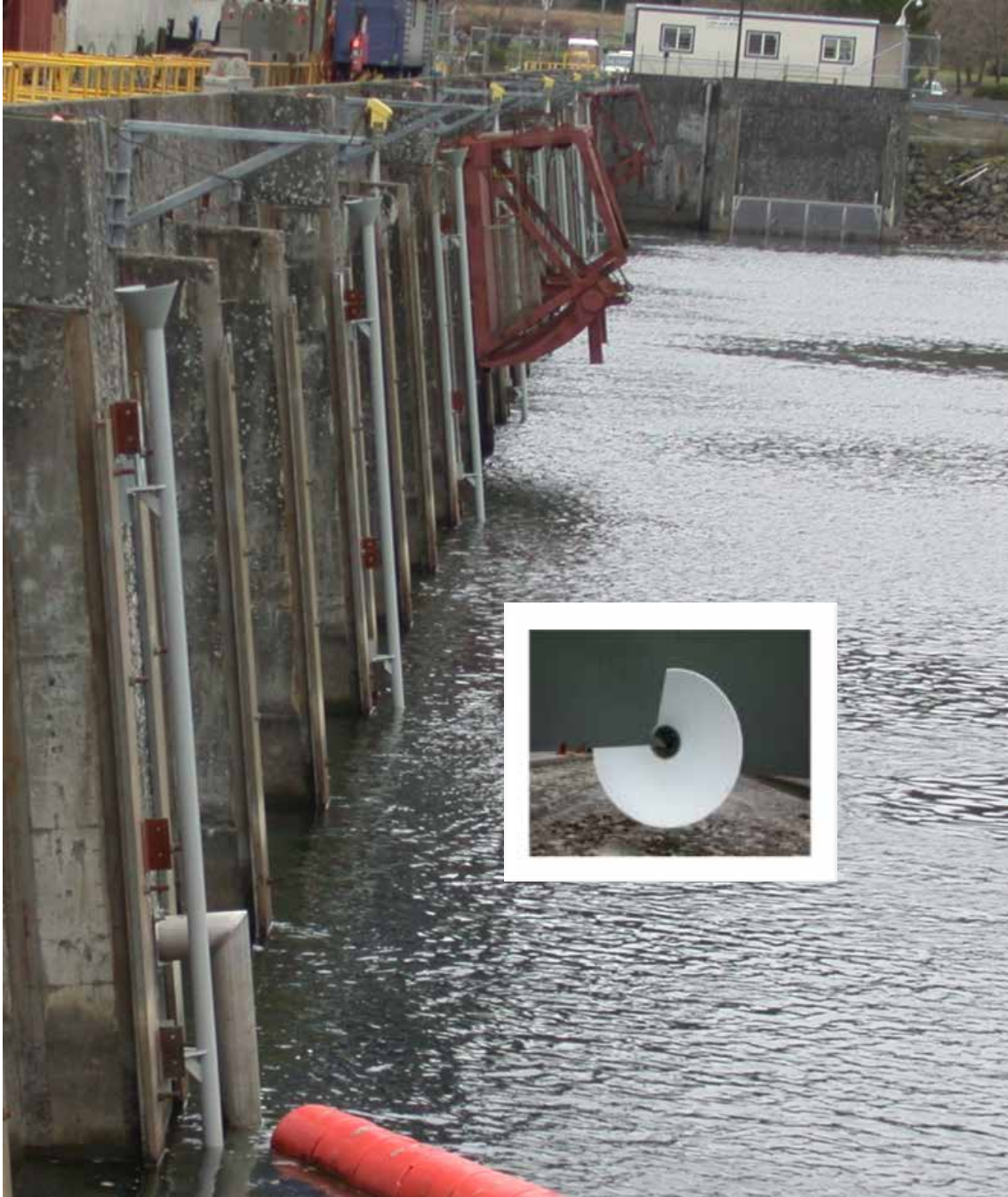
Figure 2.7. Four-Inch-Diameter Trolley Pipe Mounted on Piers at B2 (upper inset view of pipe top). Similar 4-in.-diameter pipes were installed at B1.
