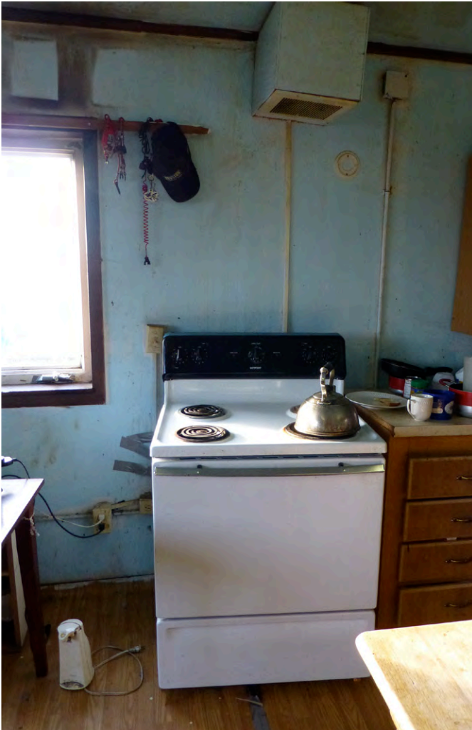
Ventilation fan installed above stove.
