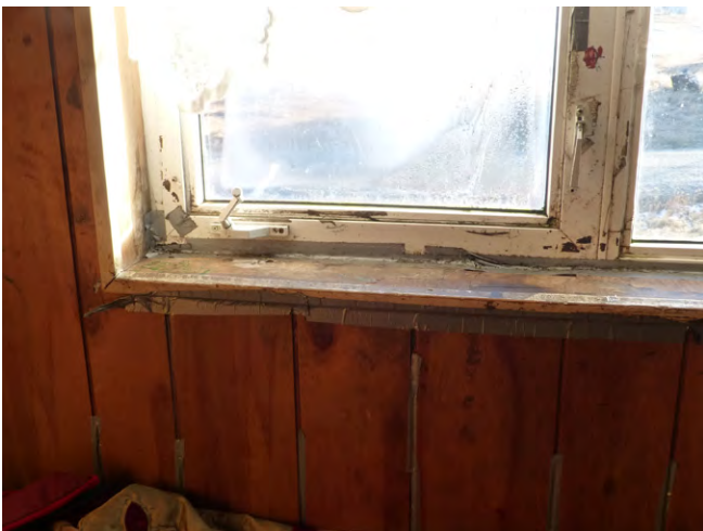
Moses Night House. Windows exhibit air leakage and condensation.
