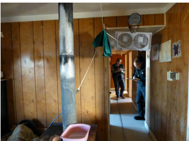
Moses Night House. Occupant has disabled ventilation system but moves warm air through house with fans.
