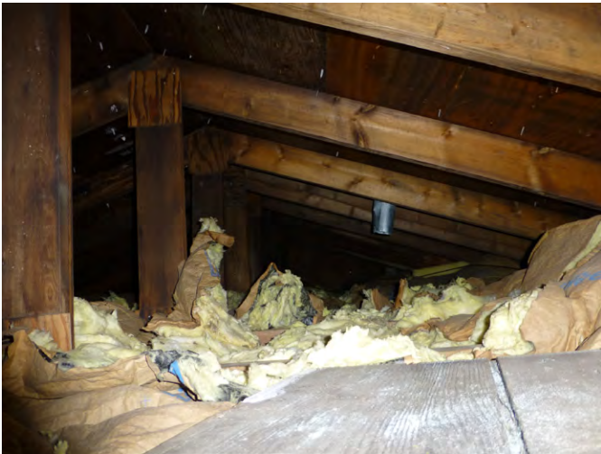
The attic hatch has no seal and is not insulated above the hatch.
