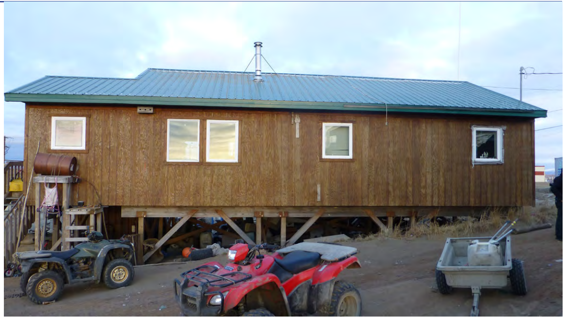
The house has experienced some settlement, but the foundation is not adjustable by occupant.
