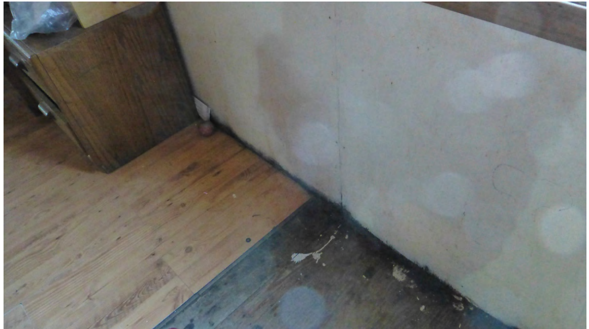
Exterior walls exhibit mold and rot at floor connection.
