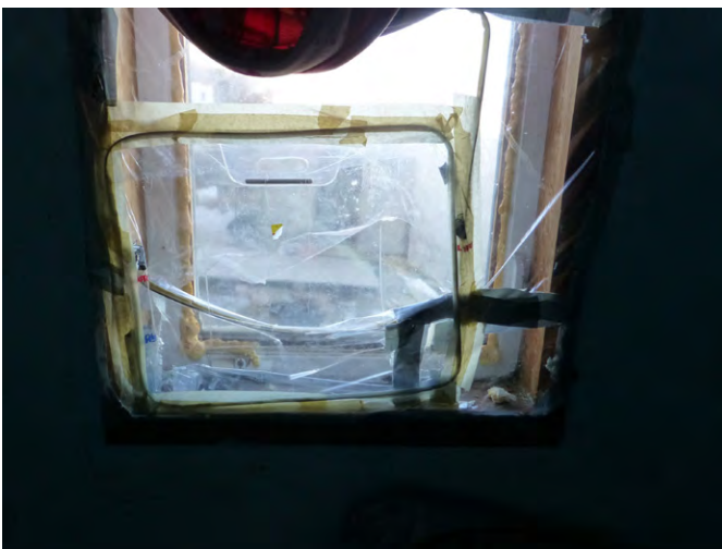
The windows are poorly caulked and drafty. The occupant covers them with plastic in the winters.
