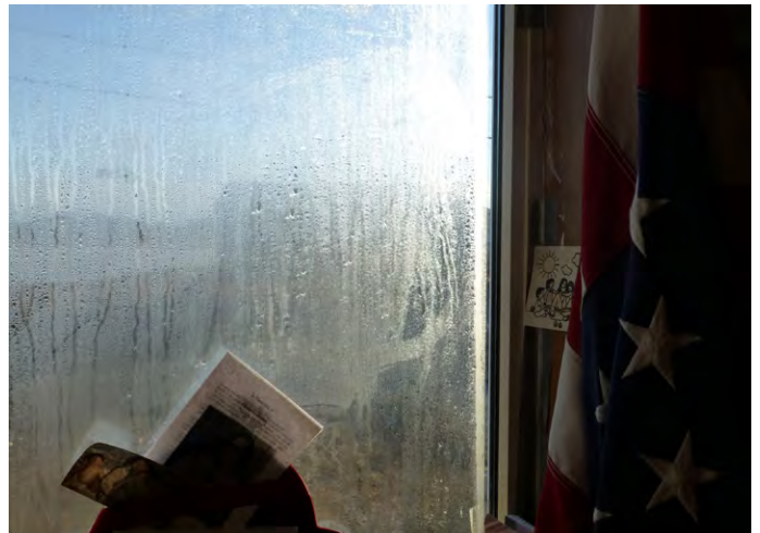
Moses Night House. Windows exhibit air leakage and condensation.
