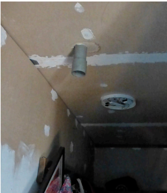
Henrietta Naneng House. A traditional passive vent has been installed in the closet for moist stale air to exit. The building depends on make-up air from the inherent lack of airtightness in the home.
