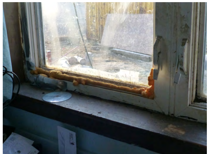
The windows are poorly caulked and drafty. The occupant covers them with plastic in the winters.
