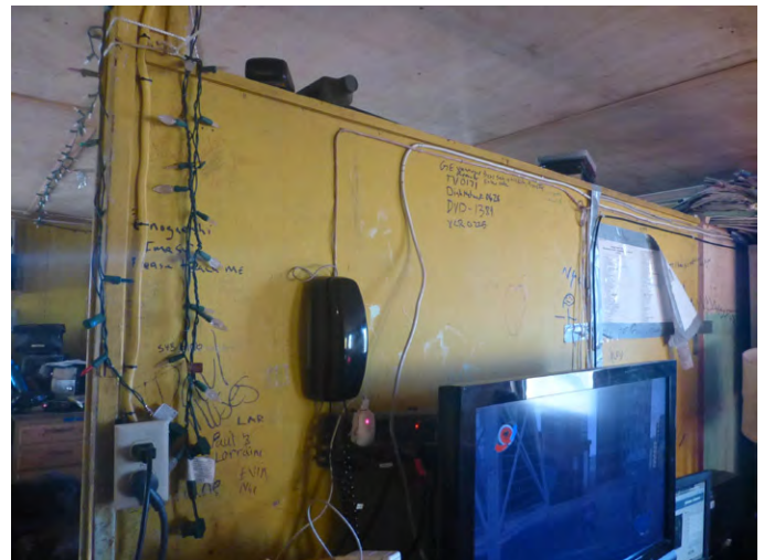
Interior walls are cut short of floor and ceilings to allow heat to move from room to room.
