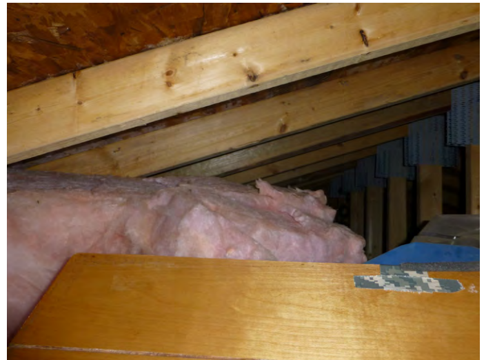
The cold roof with 8" of bat insulation and hatch into main living area
