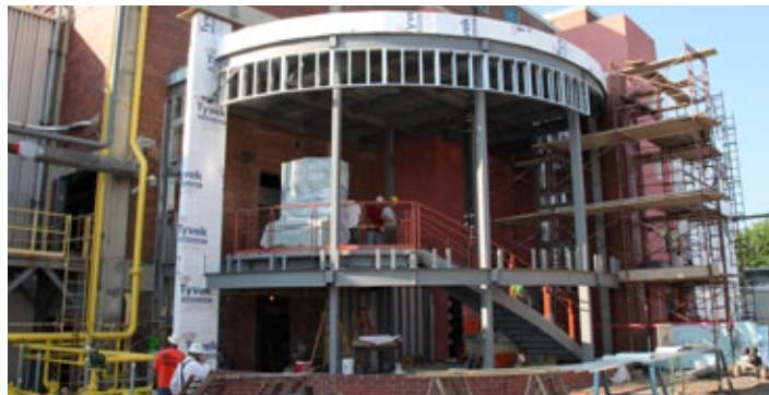
Biomass Steam Plant
