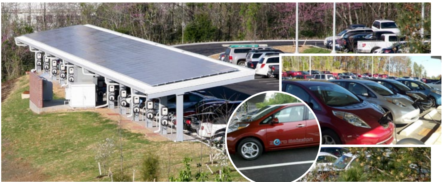
ORNL solar-assisted charging station
