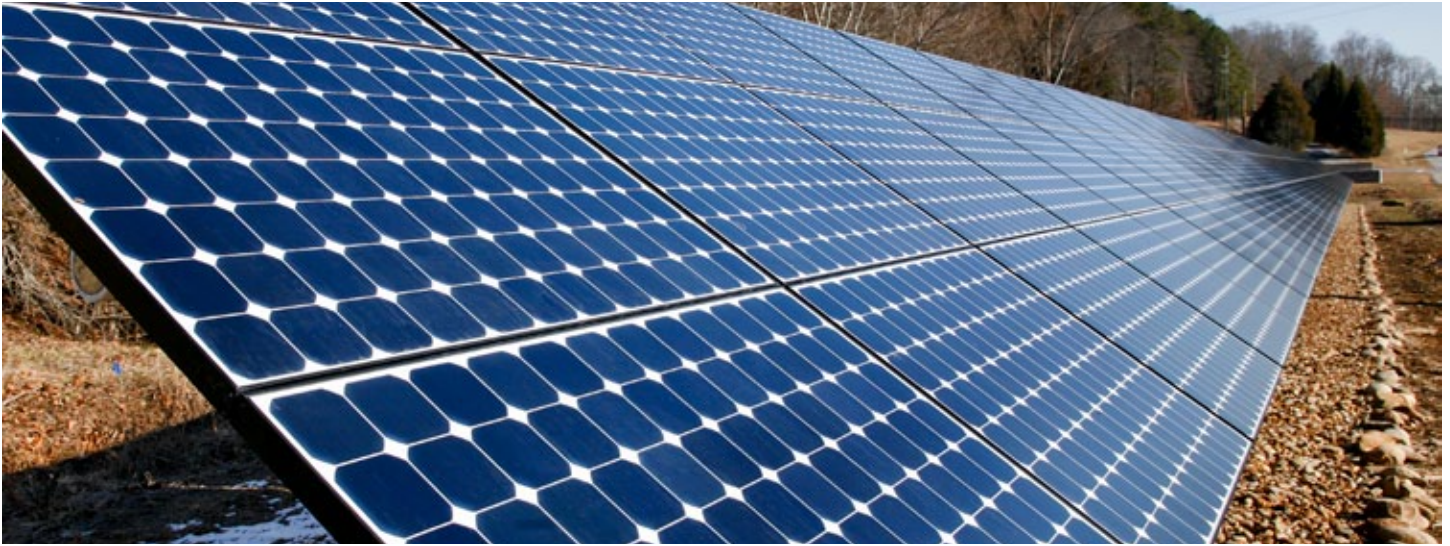
Bethel Valley Road 51.25kW Solar Array
