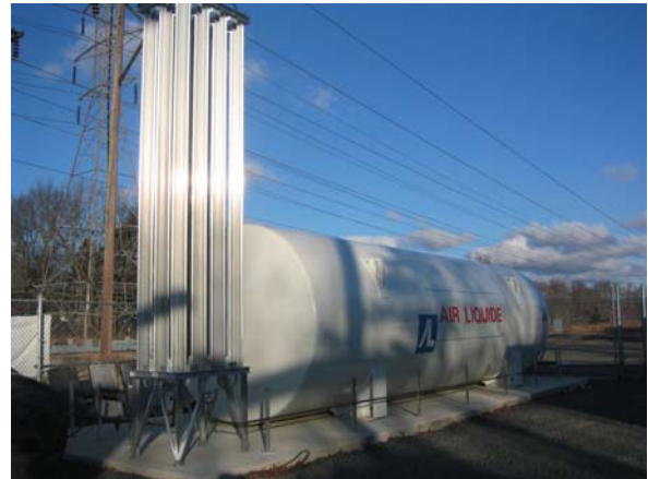
13,000 Gallon LN2 Bulk Storage tank
