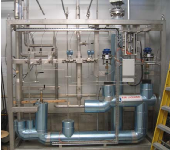
Cool Down Skid
