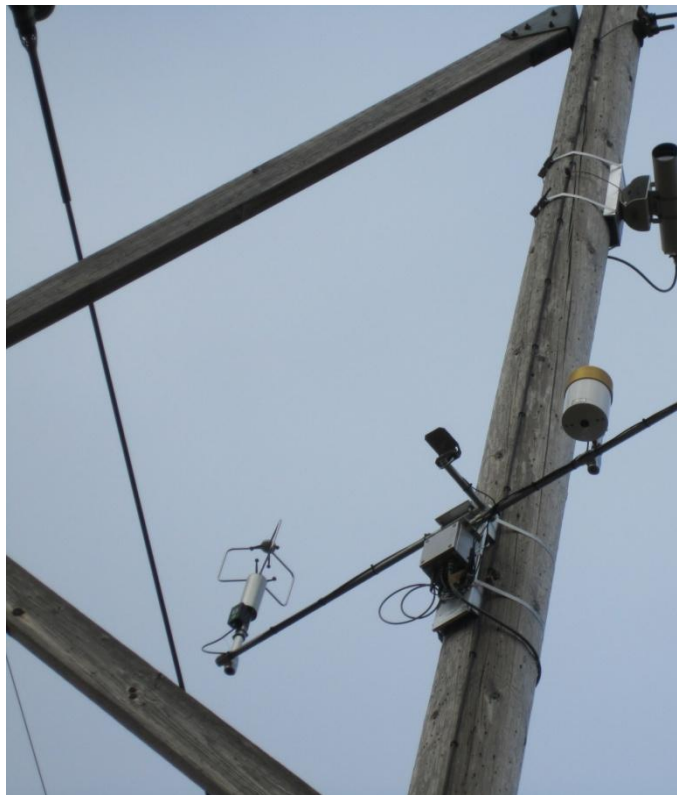
Figure D-3 Weather Station Installation at Site 3
