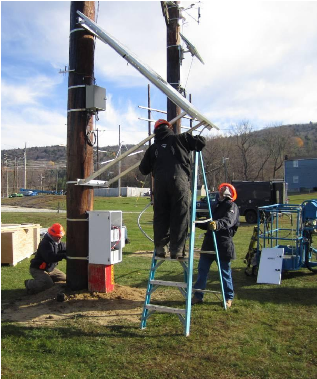
Figure C-35 ThermalRate battery box and solar panel
