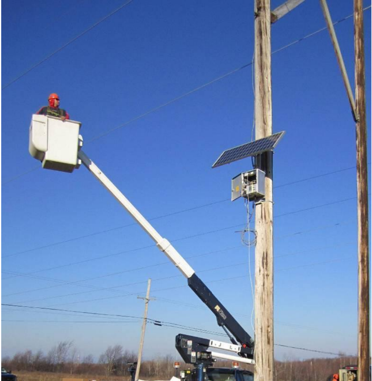
Figure C-50 Sagometer Electronic Box and Solar Panel Being Checked After Installation
