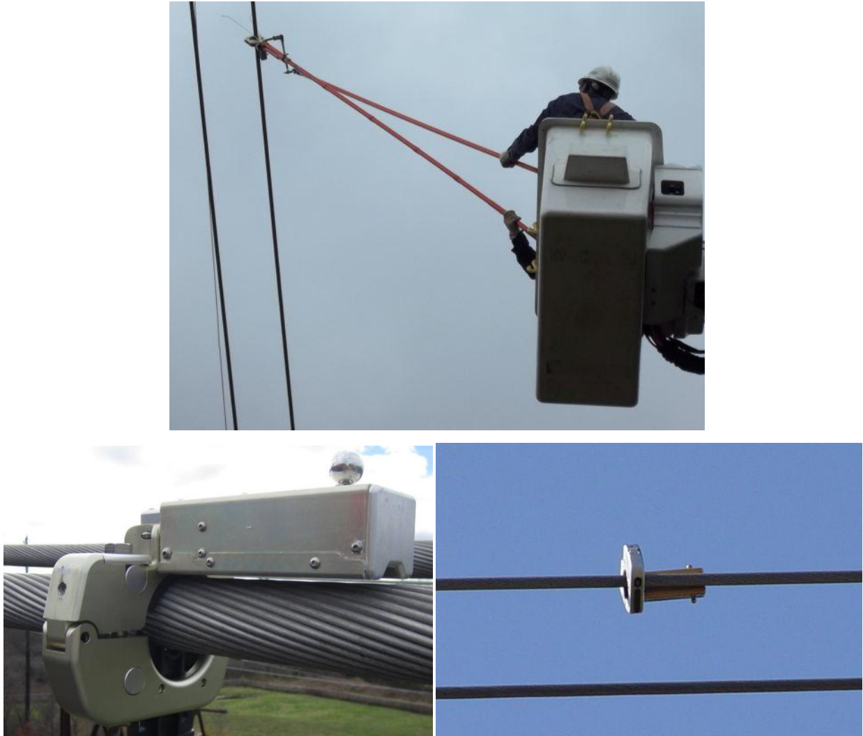
Figure C-11 EPRI Sensor installation and final mounting position on the conductor
