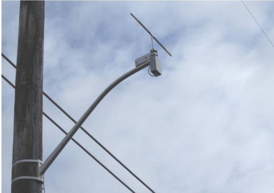
Figure C-33 ThermalRate sensor installed
