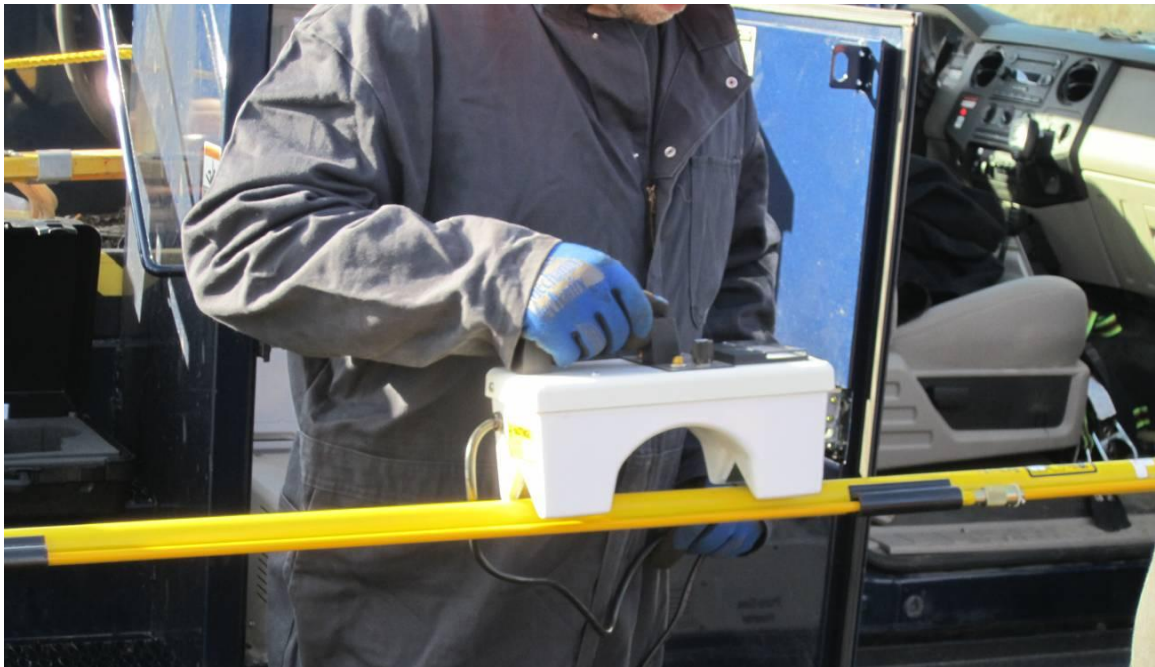
Figure C-41 Lineman tests hot stick prior to installing the EPRI Sensors on the energized 230 kV line
