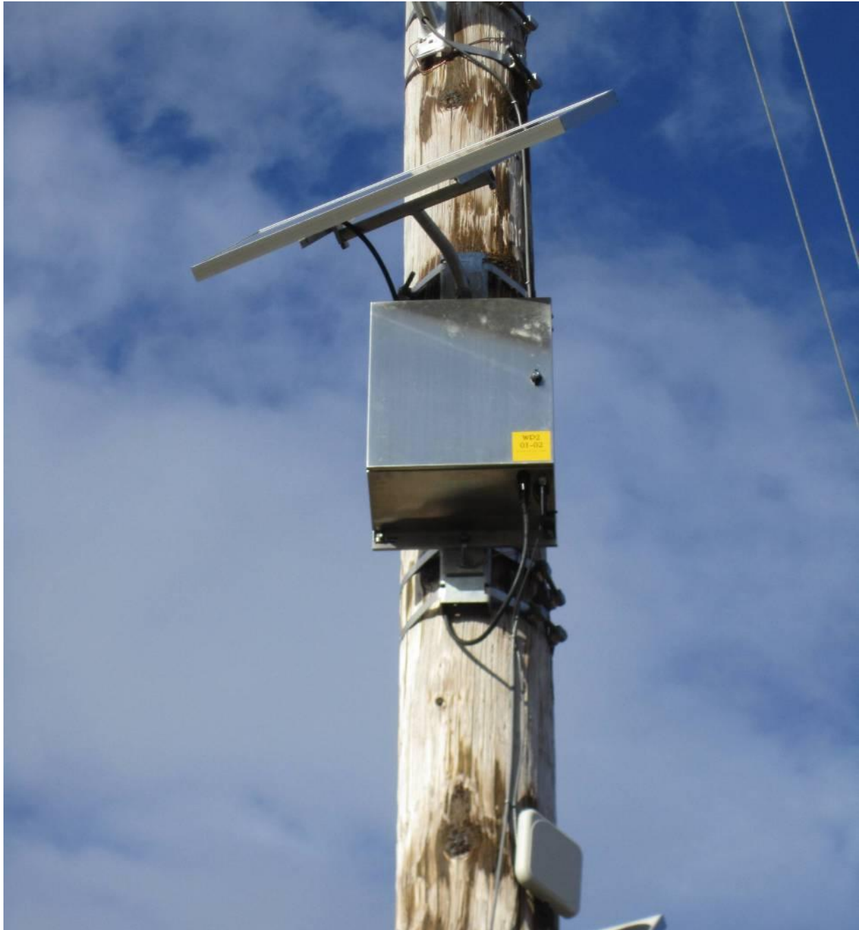
Figure C-44 EPIR Sensor electronics box and solar panel installed
