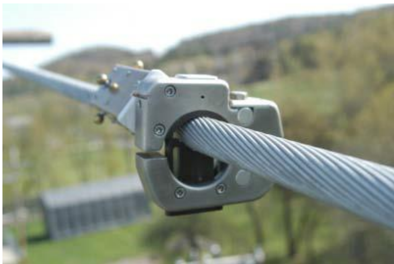
Figure G-7 EPRI Sensor Temperature Monitor
