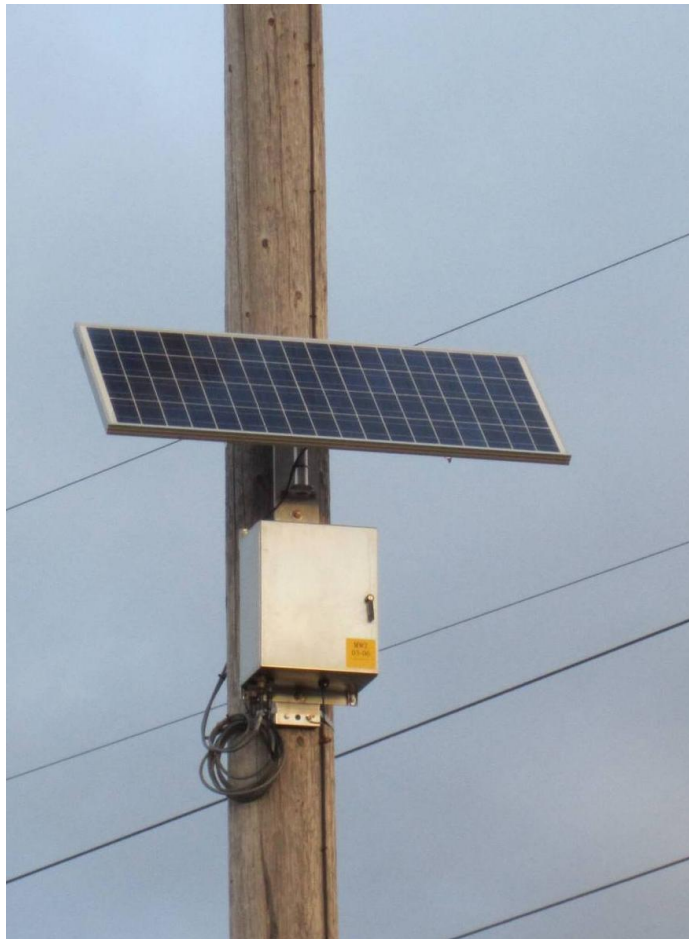
Figure C-70 Sagometer Solar Panel and Electronics Box
