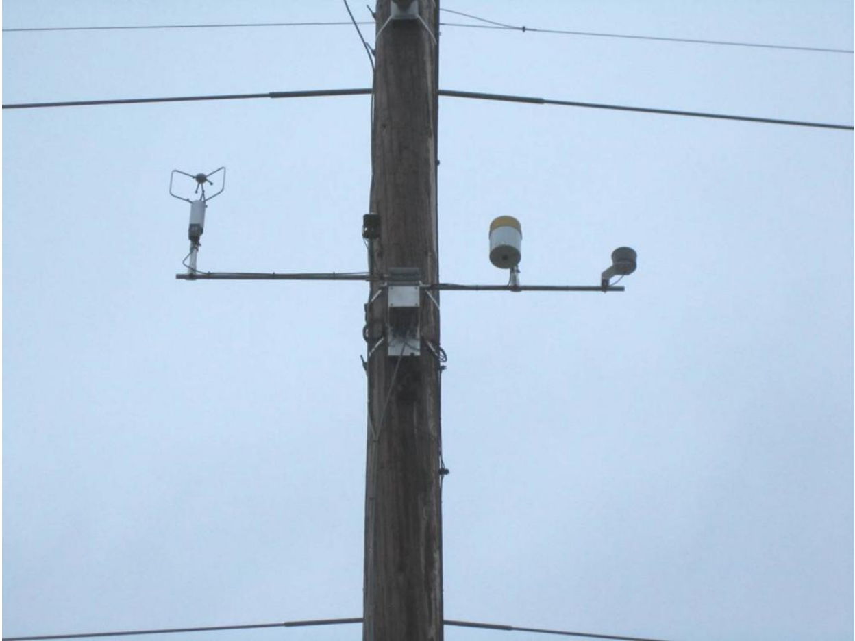
Figure C-62 Sagometer Weather Instruments Installed
