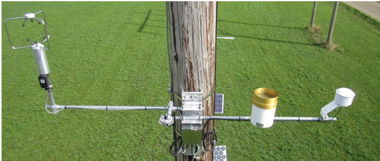
Figure C-3 Weather Station Array – left to right: anemometer, pyranometer, rain gauge, temperature/humidity sensor
