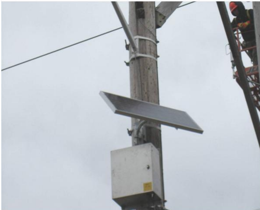
Figure C-66 EPRI Sensor Electronics Box and Solar Panel
