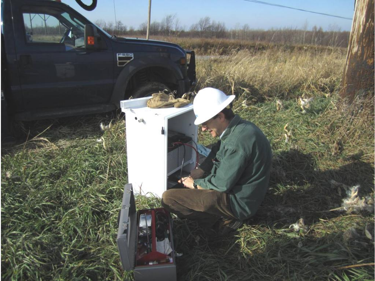
Figure C-47 ThermalRate Battery Box Being Wired
