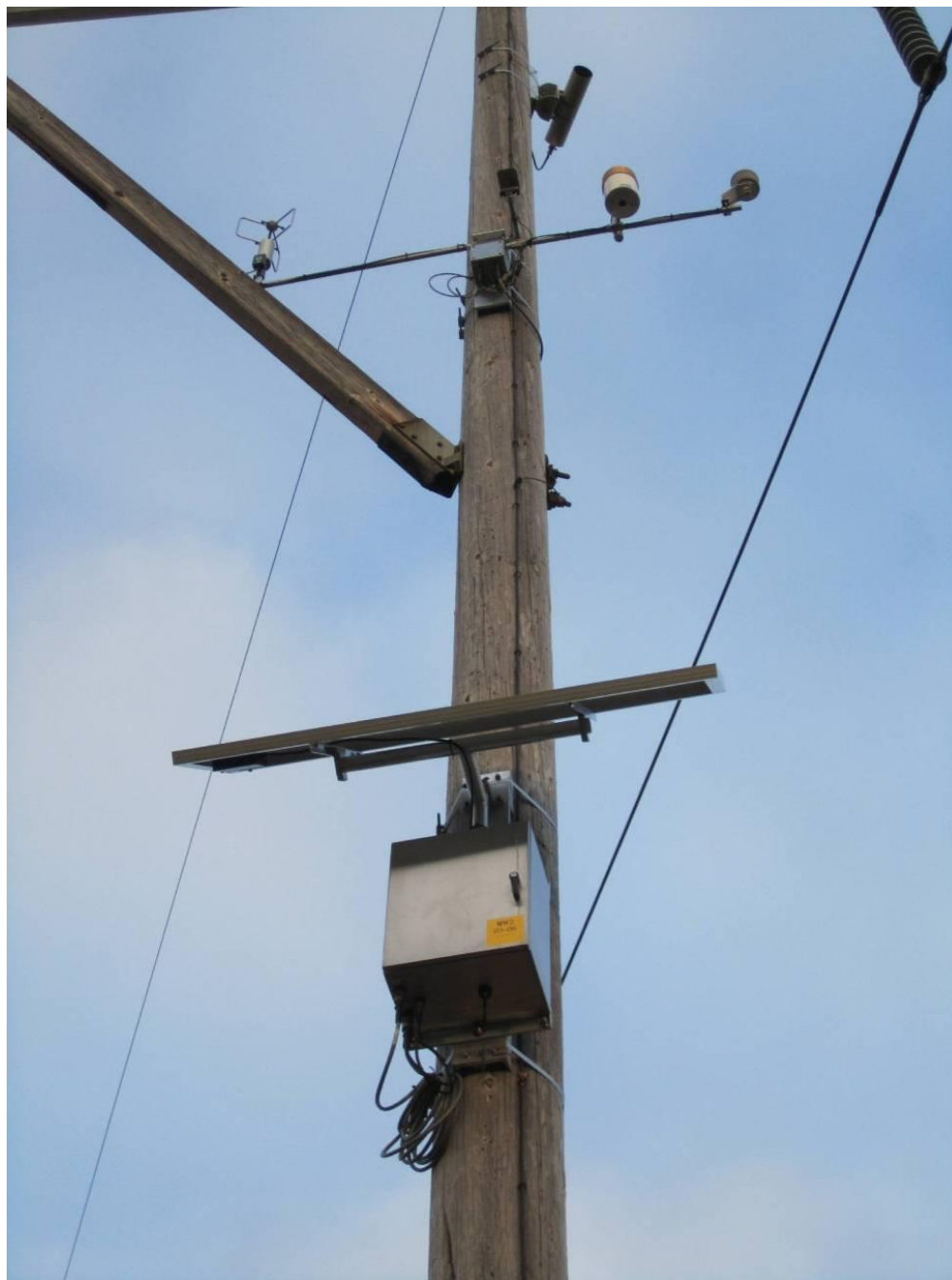
Figure C-71 Sagometer Camera, Weather Sensors, Solar Panel and Electronics Box
