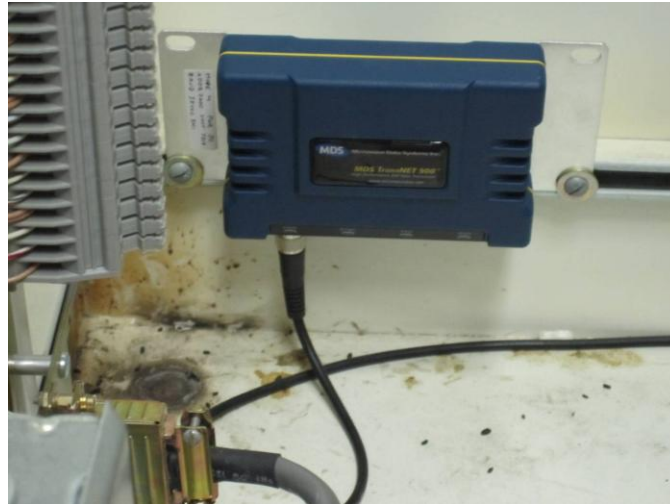
Figure C-15 Radio communication link (MDS TransNet 900) for ThermalRate System
