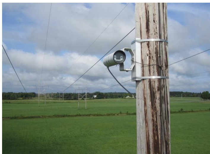
Figure C-10 Camera unit installed showing the front of the camera – The laser target illumination is mounted inside the camera unit
