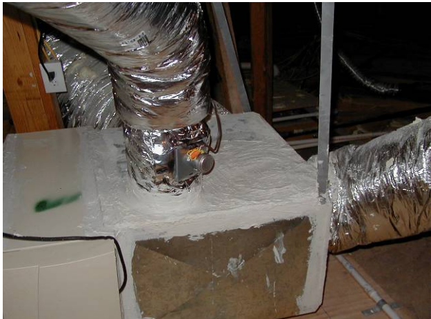
Figure 28. 6 in. Normally Closed 24V motorized damper installed
