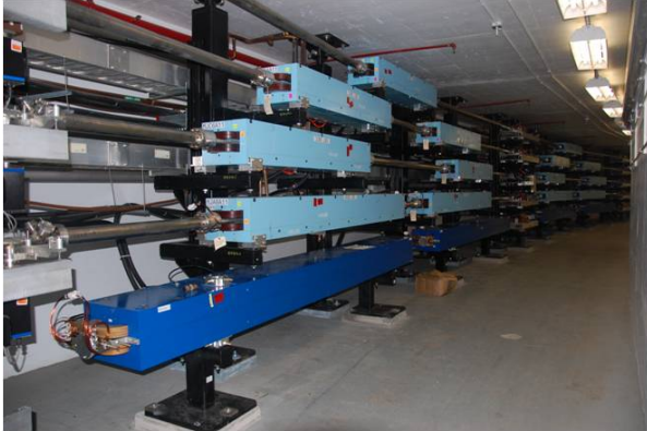
Figure 7: Re-worked and new magnets in the West Arc.
