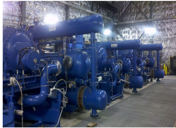
Figure 8: CHL-2 compressors are installed and are being commissioned.
