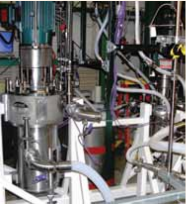
Full-scale contactors with associated pumps, tanks, piping, and an integrated coalescer in the SRNL EDL
