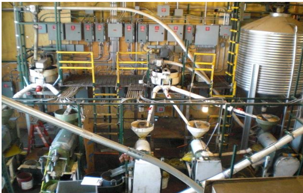
Task B.5 with view of seed conditioner, Flex-flo auger, seed chutes and electricals
