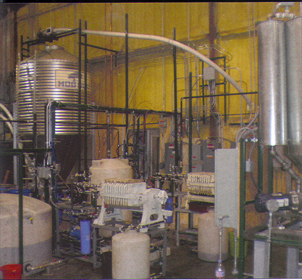
The plant, piecemealed together by county employees from 2003 to 2009, is now in operation. The next phase is to automate it, including the crush operation.
