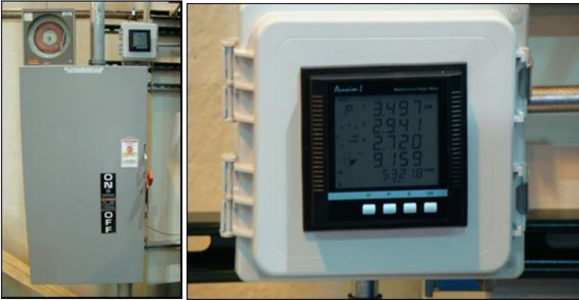
Figure 4.2.2.1-1. A. Acuvim Unit mounted on Brötje power panel. B. Close up of the front panel display of the unit.
