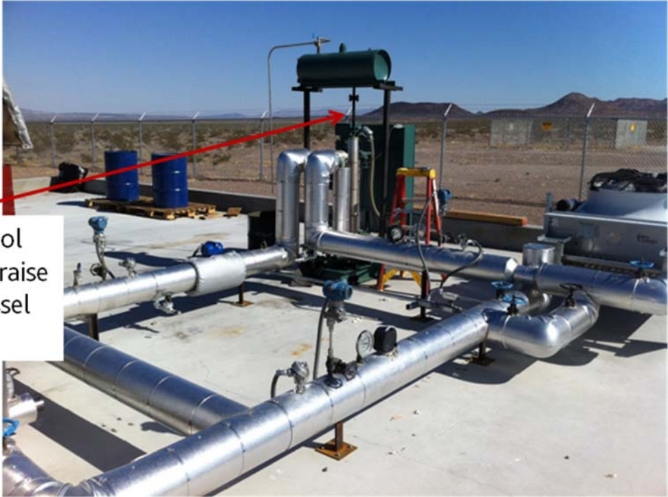
Figure 24 – Expansion vessel elevation after test loop modifications.
