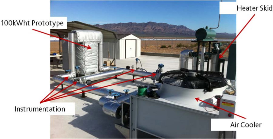
Figure 19 – Second angle of the test loop after instrumentation and insulation.
