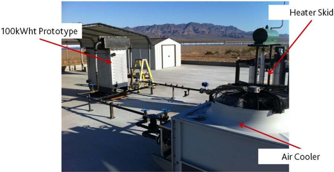
Figure 18 – Another angle of the test loop before instrumentation and insulation.
