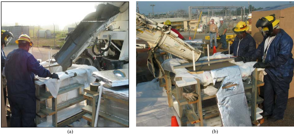
Figure 2-4. (a) Bulk tank fill grout placed into the semi adiabatic form and (b) Near full form.
