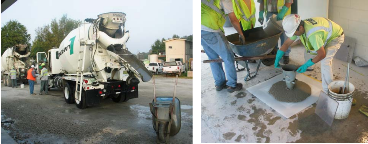
Figure 2-2. Admixture dose adjustment at the LaFarge batch plant based on ASTM C1611 test results.
