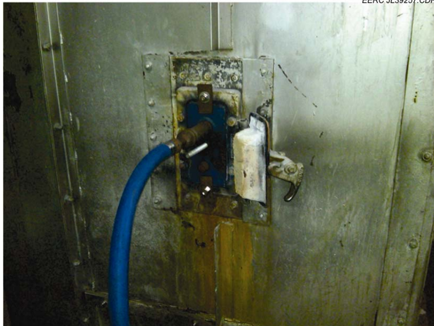
Figure 7. Modified furnace door showing injection lance installed at the northwestern corner of the boiler, fourth-floor level.
