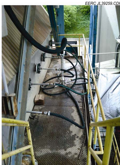
Figure 8. Sorbent injection lances located upstream of the AH. The distribution manifold can be seen connected to the main delivery line (black hose).
