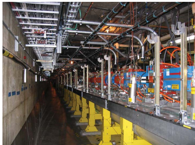
Figure 4: Sector 20 with the new FACET magnets installed.
