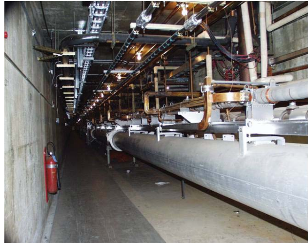
Figure 3: Sector 20 before the accelerator systems were removed to make way for FACET. The linac is visible above the much larger alignment light pipe.
