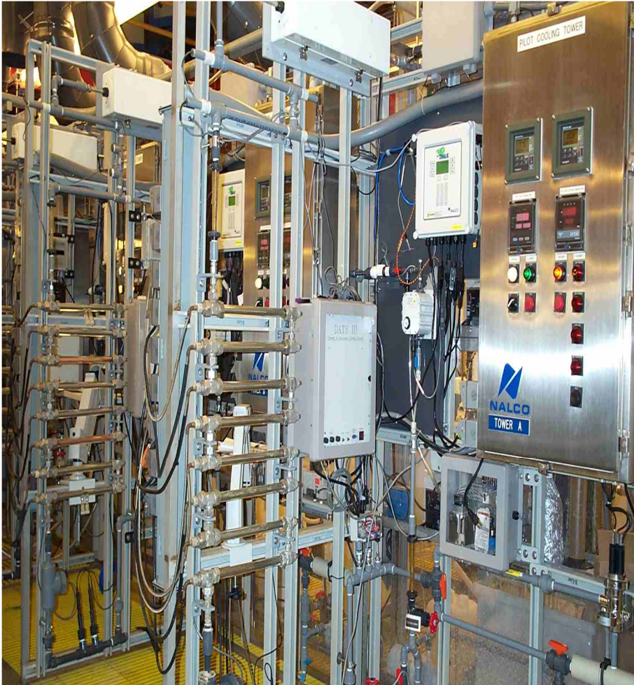
Figure 3. Pilot Cooling Tower (PCT)
