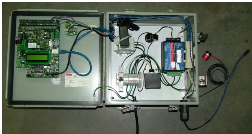
Figure 5.17. Outdoor enclosure with the sensing equipment instrumentation package.
