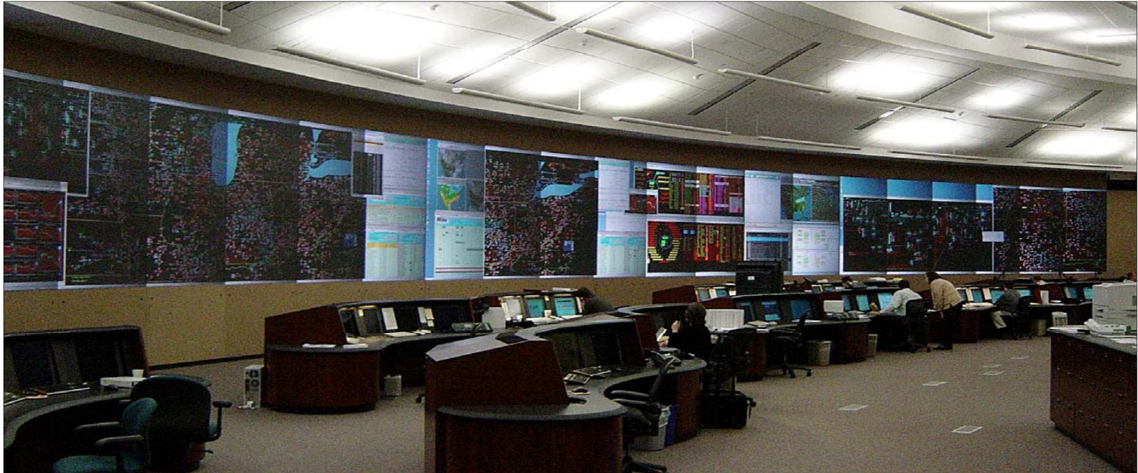
The Midwest ISO Control Room
