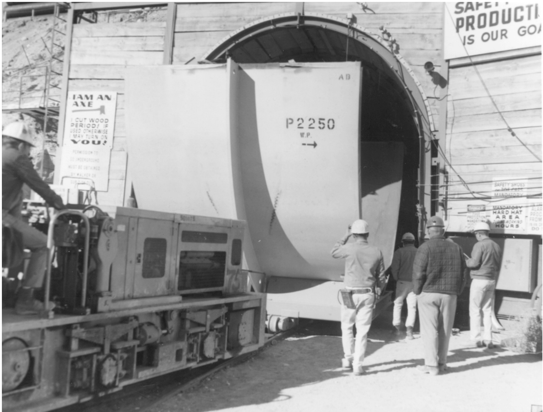
Figure 156. Half section of the line-of-sight pipe being moved into the portal entrance, U12t Tunnel, 1970 (photograph on file, Defense Threat Reduction Information Analysis Center, Albuquerque).
