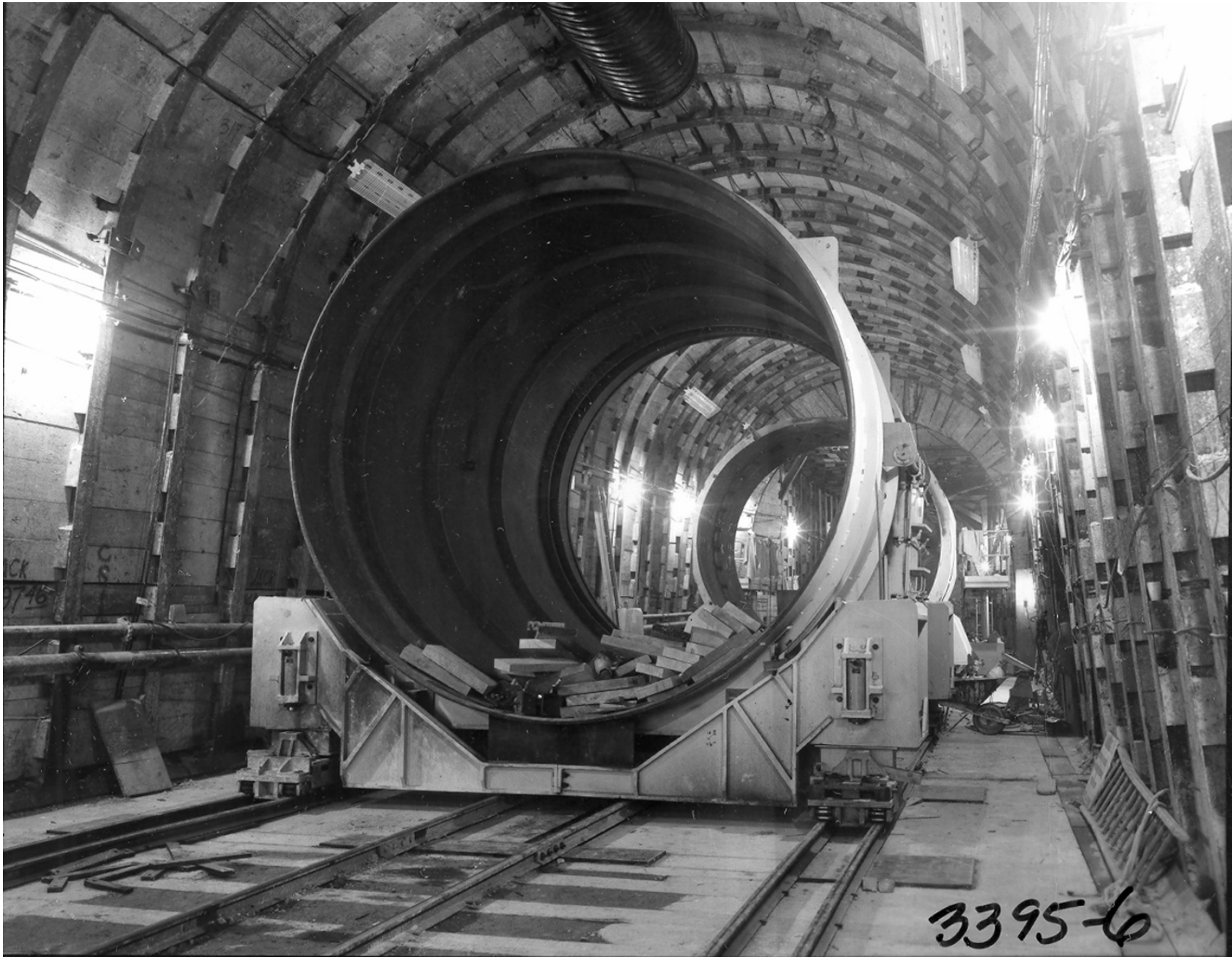
Figure 158. Construction of the line-of-sight pipe, U12t.02 drift, 1971 (photograph on file, Nuclear Testing Archive, Las Vegas).
