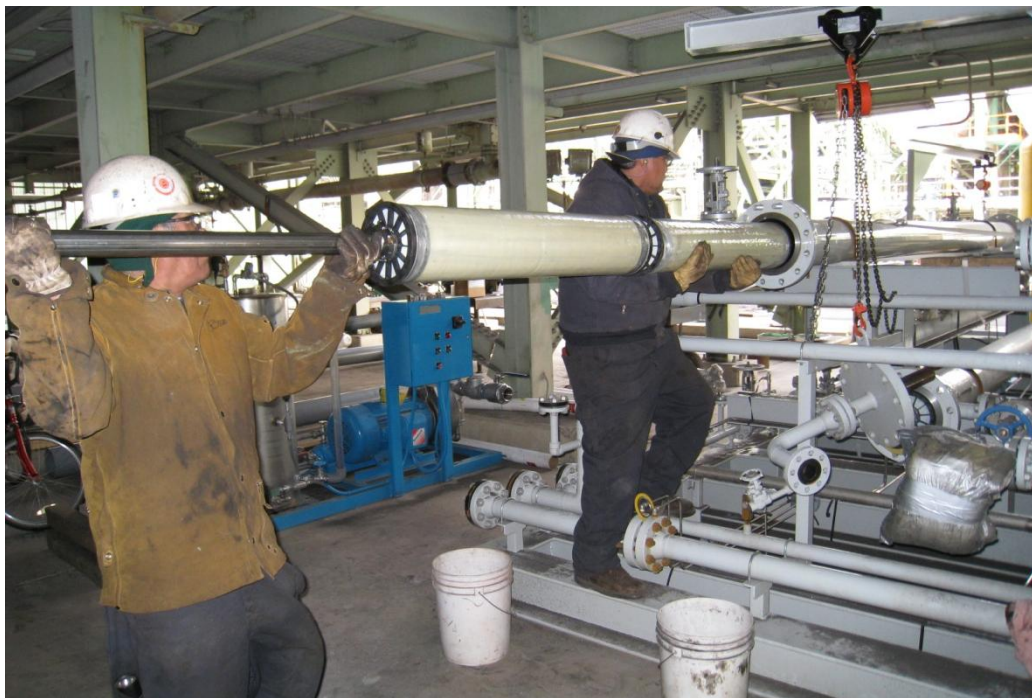
Figure 18. A picture of the 8-inch diameter Polaris modules being installed in the membrane test system at Cholla.
