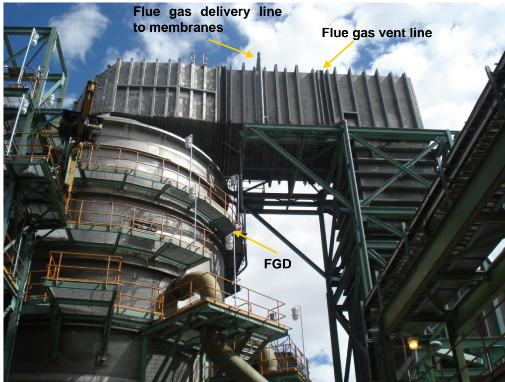
Figure 15. Photo of post-FGD flue gas line at Cholla, showing delivery line installed for flue gas delivery to the MTR membrane test skid.
