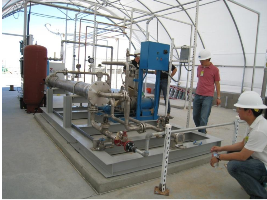
Figure 13. Photograph of the MTR Polaris™ membrane skid for capturing CO 2 from flue gas at the APS Red Hawk natural gas-fired power plant.
