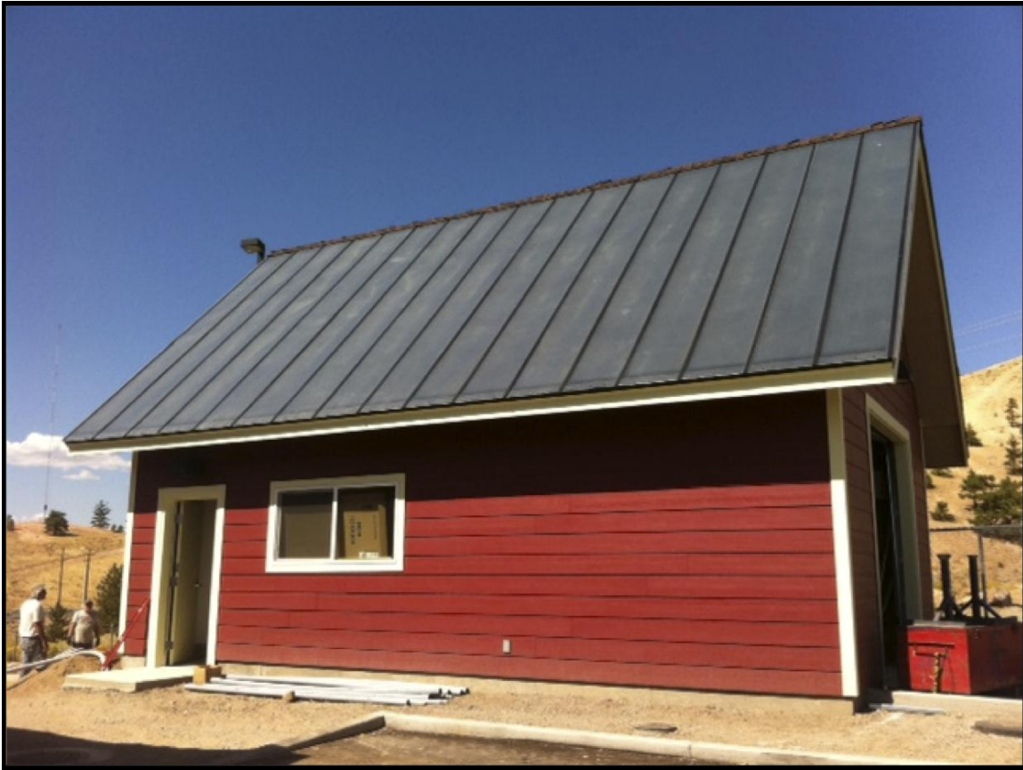
Figure 9 578 square foot (34' by 17') site-built roof-integrated solar air heater. The backside (building roof and overhangs) is insulated.
