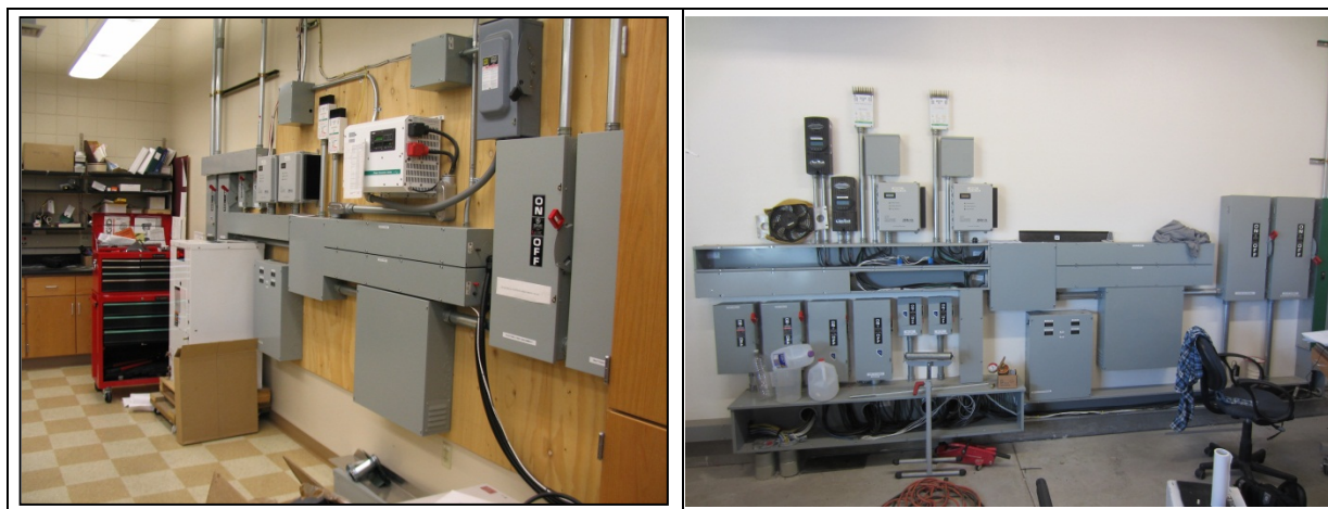
Figure 35. Moving of power monitoring and control equipment for renewable power system.
