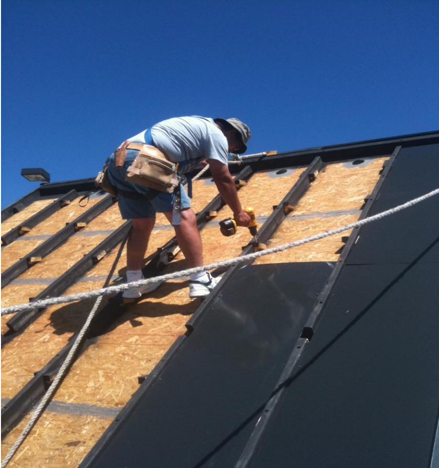
Figure 6 Black Sheet Metal Sheets are screwed onto the support blocks to become the Absorber. Air exit holes into the building are shown at the top of each bay.
