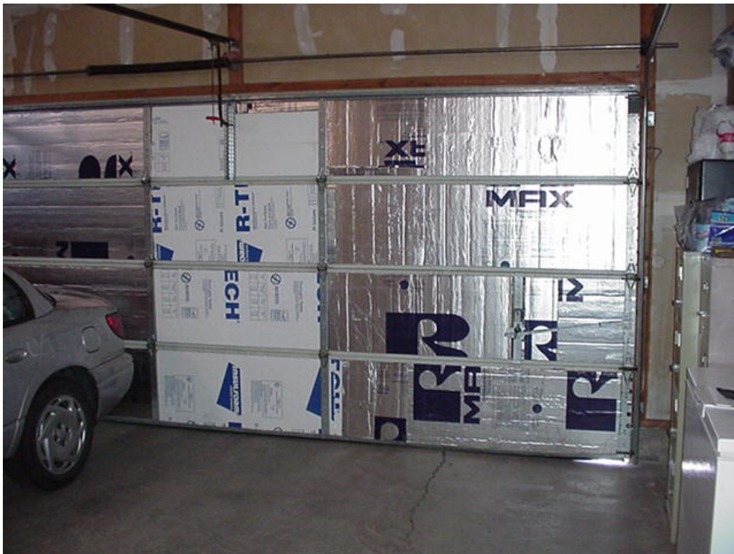
FIGURE 2 The foil-backed insulation cuts cleanly with a razor knife, whereas the compressed (white) styrofoam tended to crumble into messy electrostatic crumbs. The insulated garage is much more comfortable both winter and summer, and helps moderate the temperature of the attached living space.
