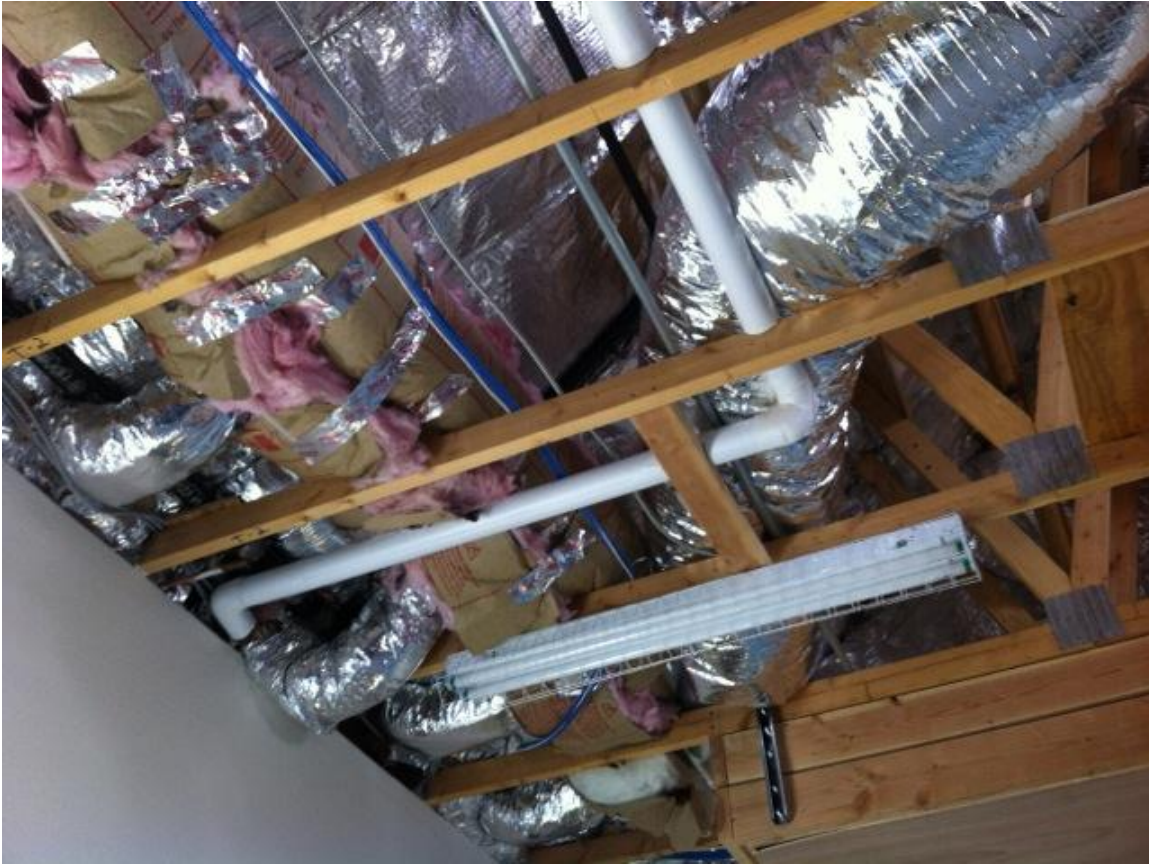
Figure 11 Each of two headers comprising the duct distribution system is connected to the solar collector through 15 sets of collars which support flexible ducting. In the upper right the silvered insulated duct from the blower connects with a 14" diameter duct which is insulated with tan exterior wrap. Insulated silvered collars connect with the collector every 2 feet. A similar header at the top delivers heated air to the heat exchanger box.
