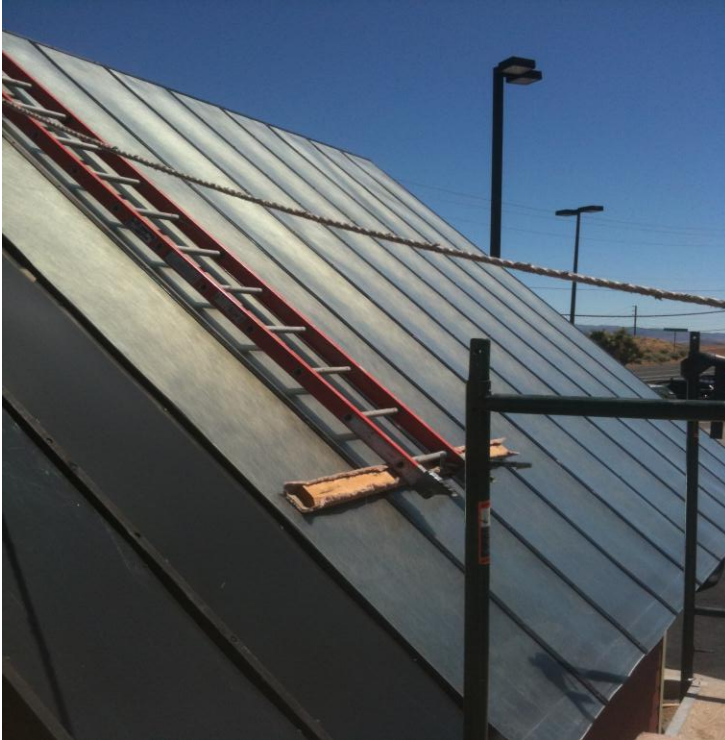
Figure 7 Glazing panels are secured by black aluminum battens. The area to the lower left awaits a glazing strip.
