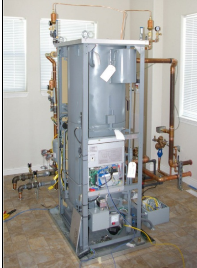
Figure 28. Yazaki absorption chiller in utility room of REEF House
