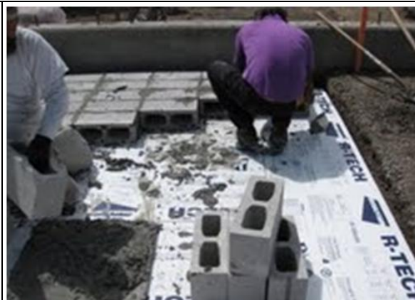
Figure 19. Holes in concrete blocks form air channels, allowing flow of heated air in winter and night-chilled air in summer.
