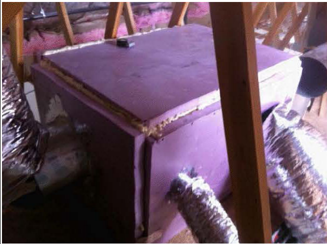
Figure 21. Insulated heat exchanger box containing three MagicAire SHW-2 2525 10 heat exchangers.
