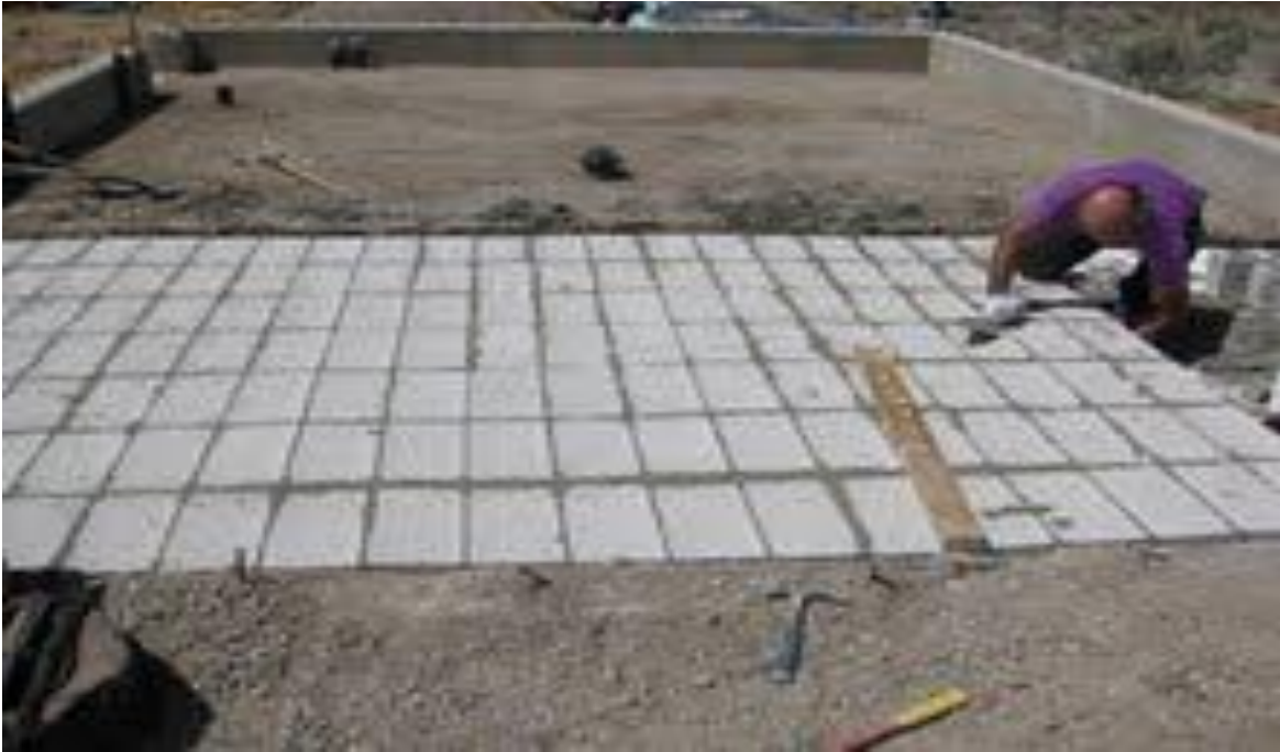
Figure 13 Hollow Concrete blocks were positioned to align holes into air channels. The blocks were sited over 2” of rigid insulation. 5’ or concrete floor were sited over the blocks. At either end headers allow air to pass through the channels. In winter, solar heated air passes through the channels, heating the concrete floor for night release. In summer evaporative cooled air passes through the hollow floor at night, storing night coolness for release the following day.
