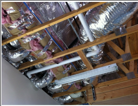
Figure 16. REEF solar thermal air system header, inside Workshop.
