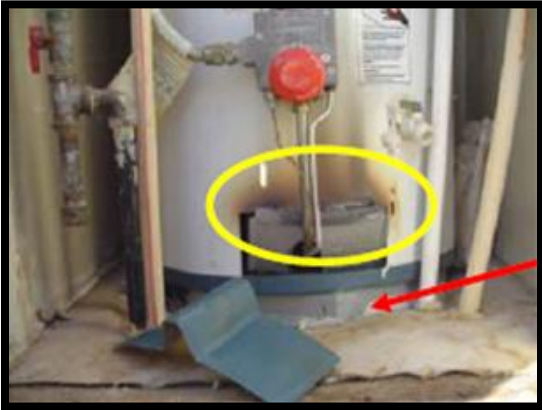
Fig. 1. DHW tank flame rollout [1].
