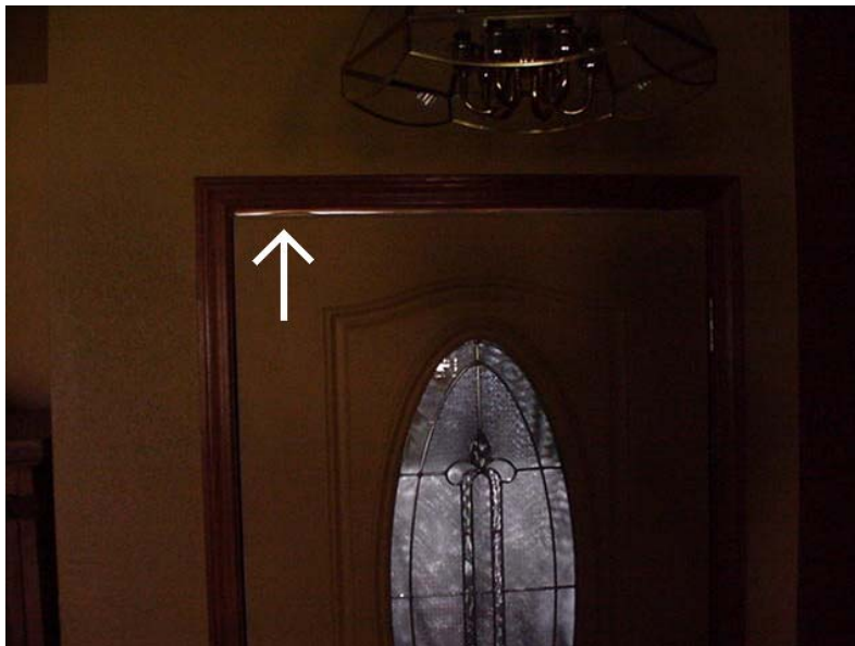
FIGURE 1 The crack above this front door will be filled in with rubber or felt weather stripping applied to the frame, or the door top, or both.
