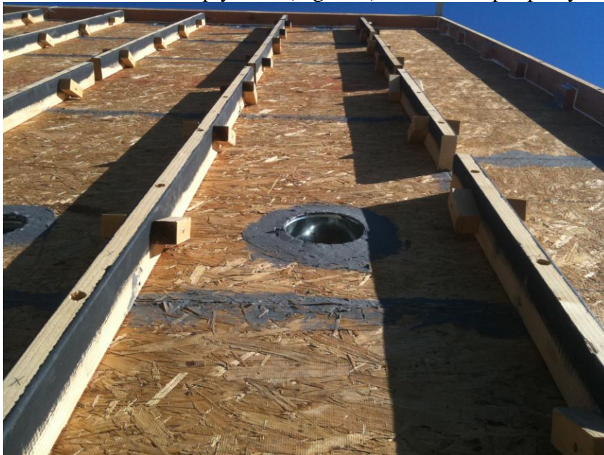
FIGURE 4 Collector Framing Detail, also showing a heavily caulked air inlet port
