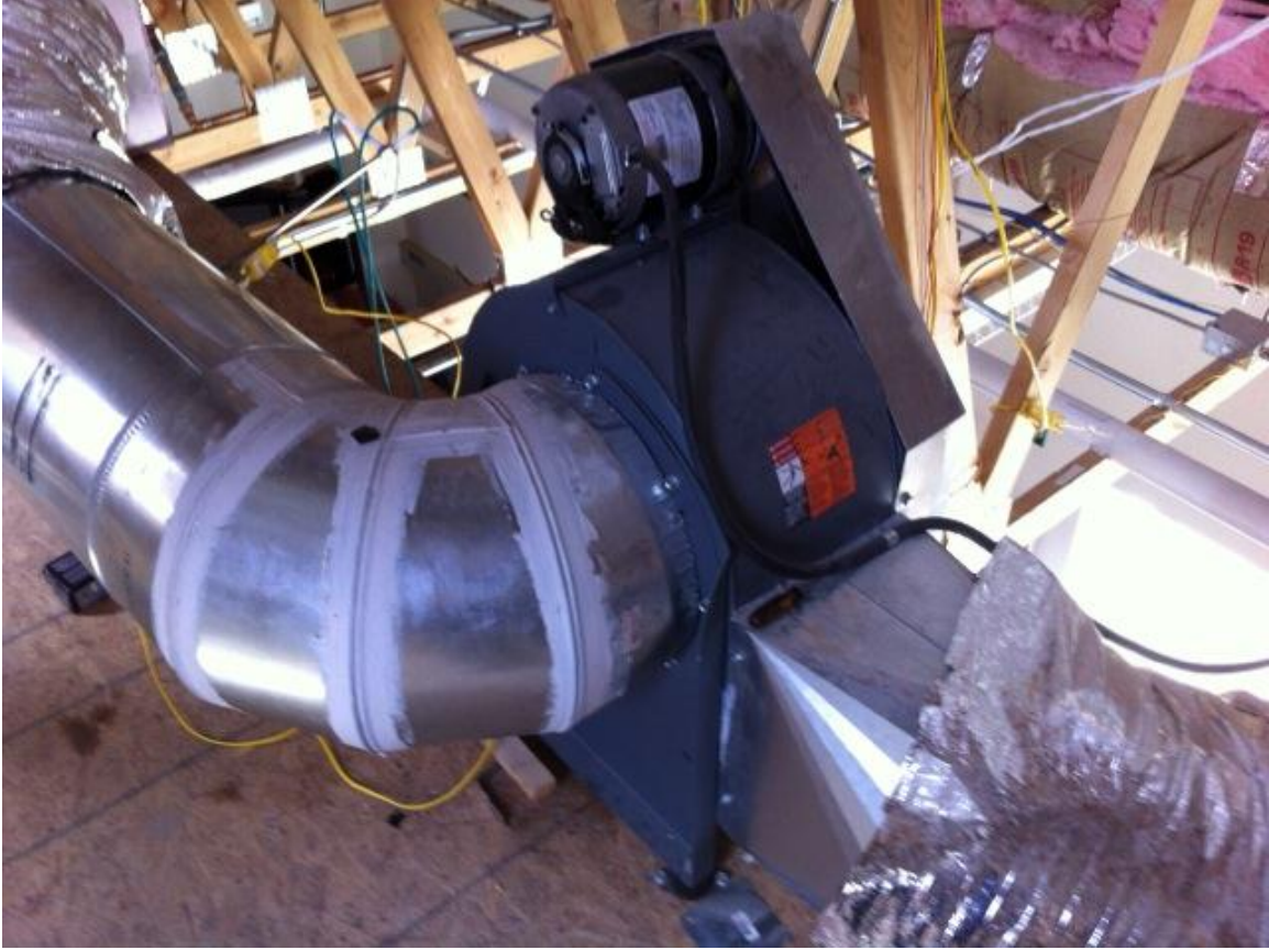
Figure 12 The 2100 cfm blower delivers air to the collector intake header.
