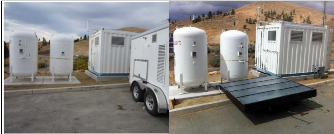
Figure 10. Electrolyzer and hydrogen storage tanks within the DRI-REEF.
