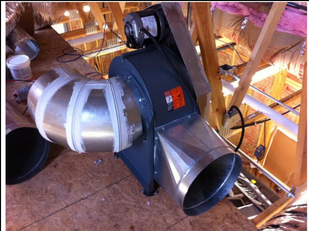
Figure 17. Dayton 7C653 2100 cfm blower within REEF Workshop delivers air to the collector intake header.
