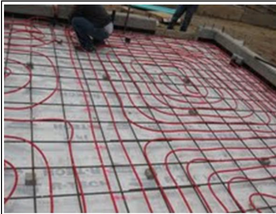
Figure 18. Water tubes placed on rebar, over 2" of rigid insulation, prior to pouring the REEF Workshop concrete floor.
