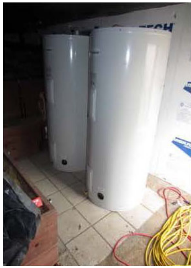
Figure 27. Water tanks for thermal storage installed under REEF House.
