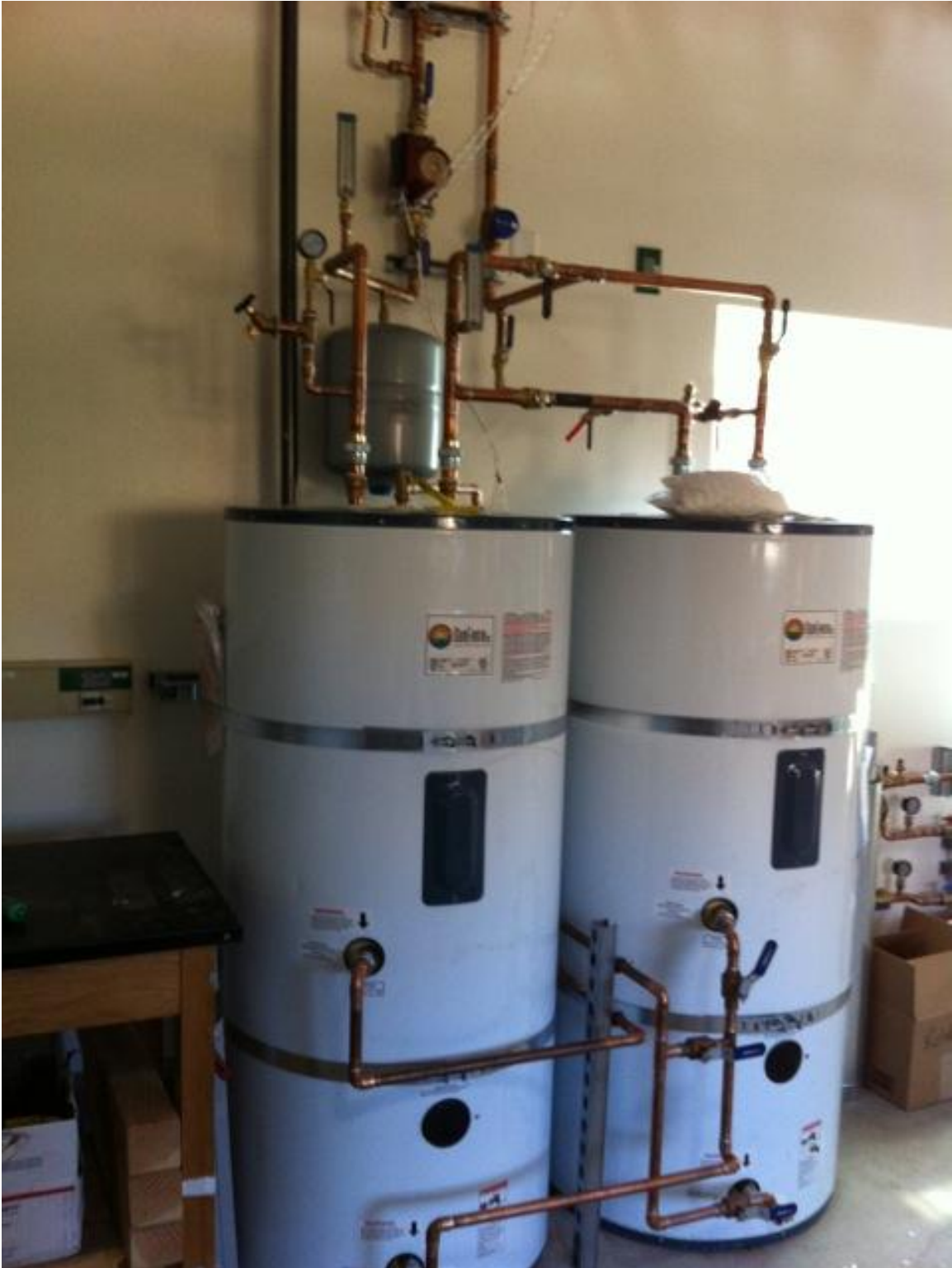
Figure 17 Twin 120 gallon water tanks store potable water under city pressure. They are connected as depicted in Figure 15. Water is circulated by the red pump (upper center)
