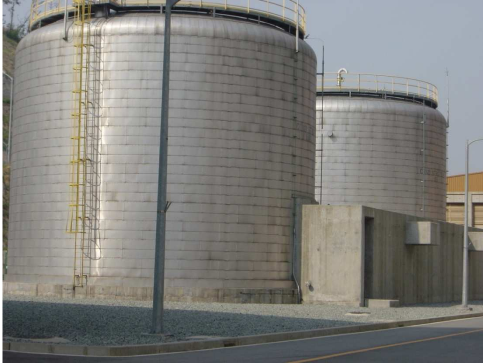
Figure 3-1 Photo of the Condensate Storage Tanks [Nie et al., 2010, 2011]
