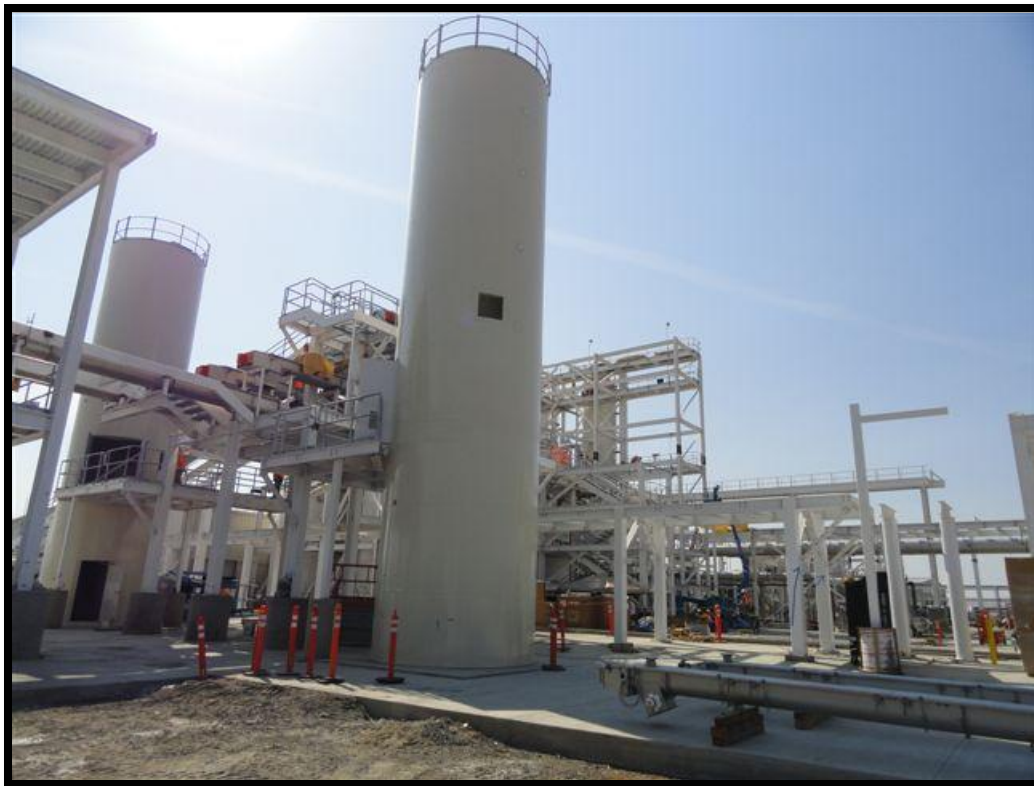
Figure 10 - 2W P&T Lime Storage Silo
