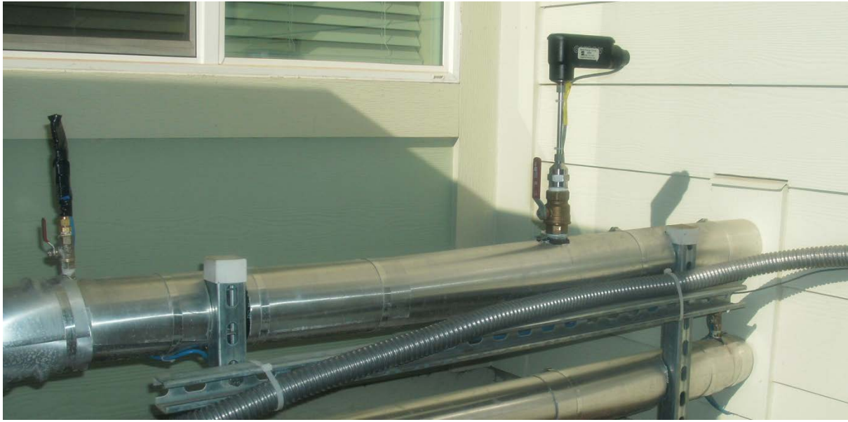
Figure 4. Flow meter installed on the hot water supply line leaving the heat pump unit
