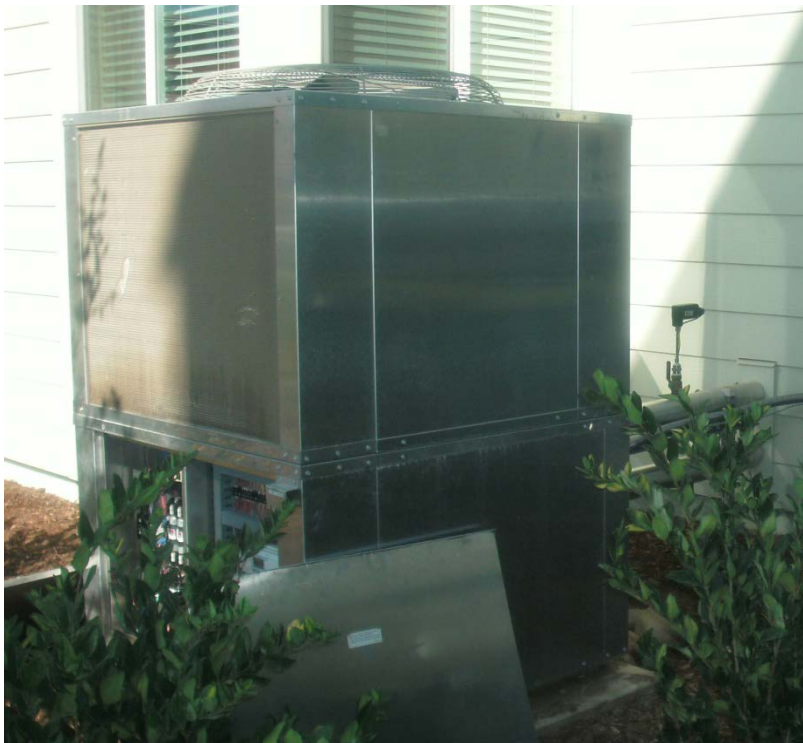
Figure 3. HPWH installed on Ramble Building #1
