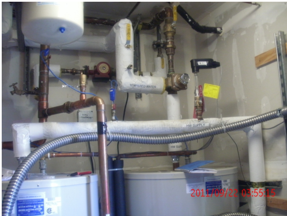
Figure 5. Two hot water storage tanks with electric resistance auxiliary heat and water piping. Flow meter and temperature sensor can be seen on the hot water supply line between the two tanks.
