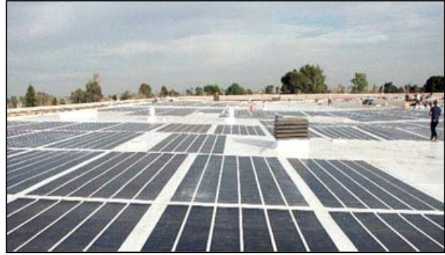
Figure E-2: Integrated PV on Rooftop
