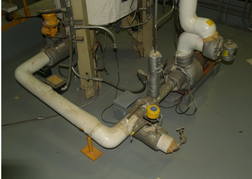
Figure 5. Sodium reaction vessel recirculation pumps and piping.
