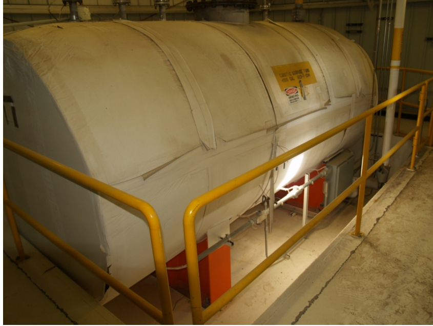
Figure 7. Caustic storage tank.
