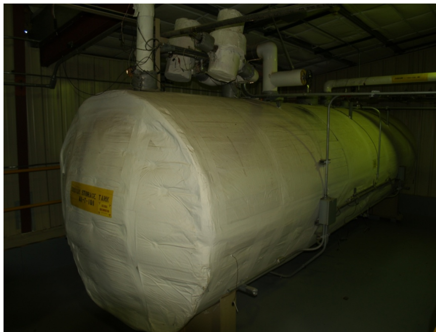
Figure 2. Sodium storage tank.
