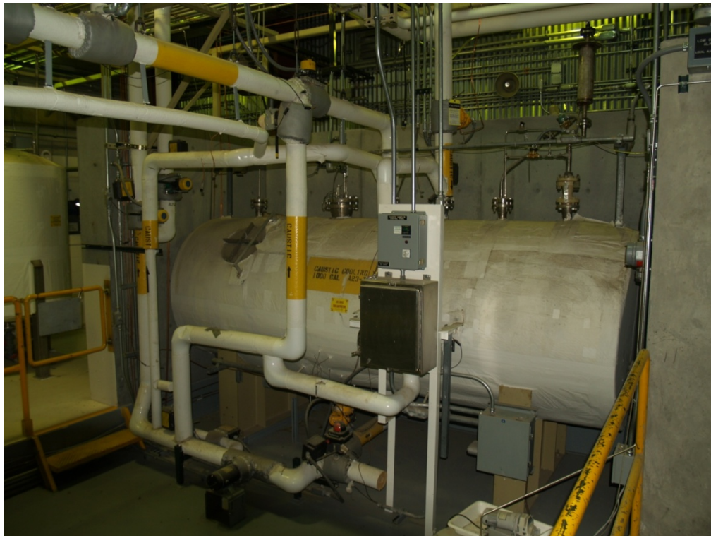
Figure 6. Caustic cooling tank.
