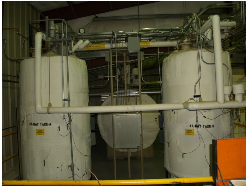
Figure 3. Sodium day tanks.
