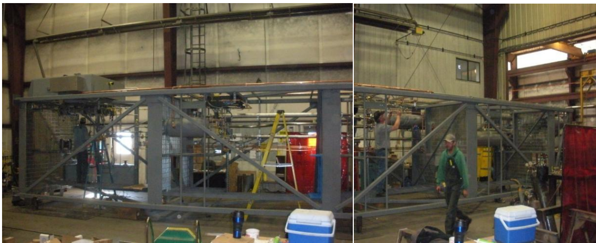
Figure 35: Picture of Tower for the 1 kW Pilot Equipment
