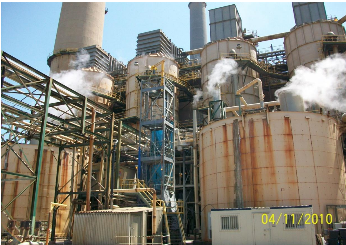
Figure 42: Picture of the 1 kW Pilot Installed at Martin Lake
