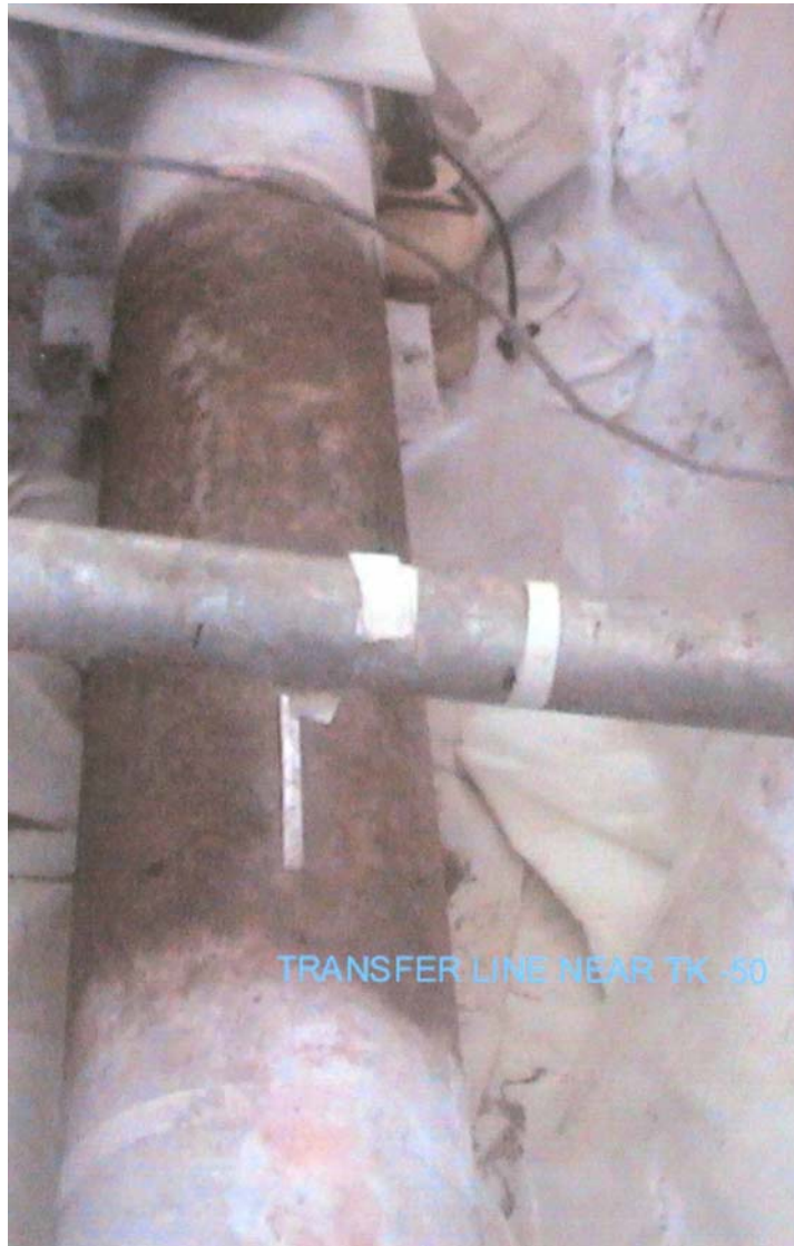
Figure 26. View of Line #1663 (near Tank 50) that shows corrosion of the exterior of the jacket [103].
