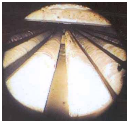
Figure 1. View of Type I Transfer Lines in Concrete Encasement between Tanks 1 to 8 in F-area
