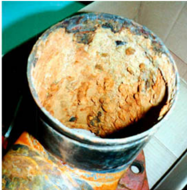
Figure 11. Microbiologically induced corrosion on a pipe [39]. Note that this is not pipping from the SRS waste transfer line system.
