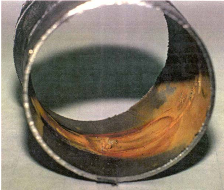
Figure 14. Dry tubercle and ring stains on pipe weld associated with MIC [67].
