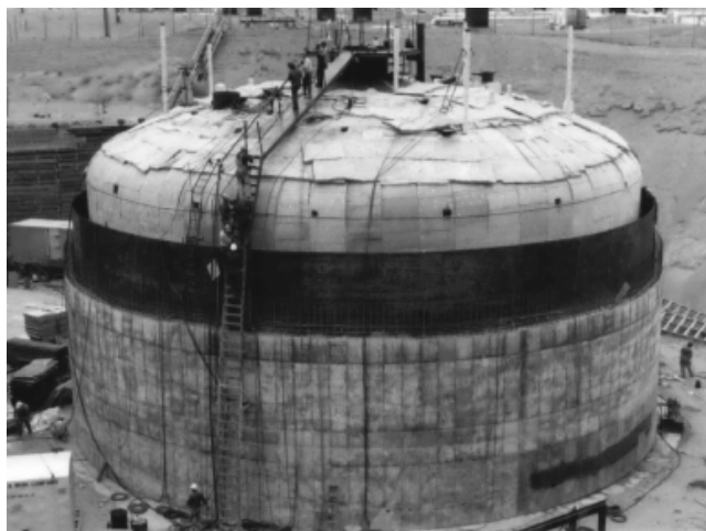
Figure 4-14. Insulation Covering the Primary Tank of SY-102 Prior to Stress Relieving (Photo 69402-39) (Taken 6-19-75)
