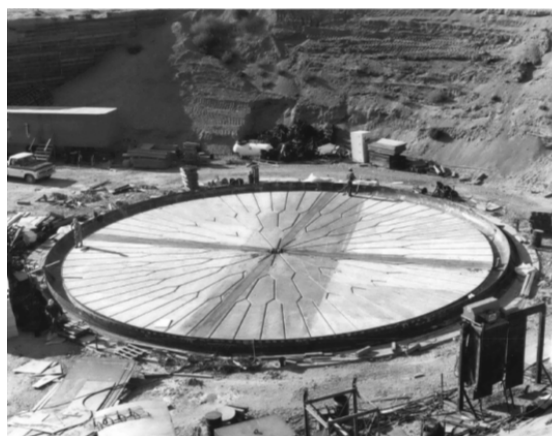
Figure 4-6. Tank 241-SY-102 with Refractory Filled in Over Air Ventilation Supply Pipes and Air Channels Cut into Refractory (Photo 66542-6) (Taken 10-22-74)
