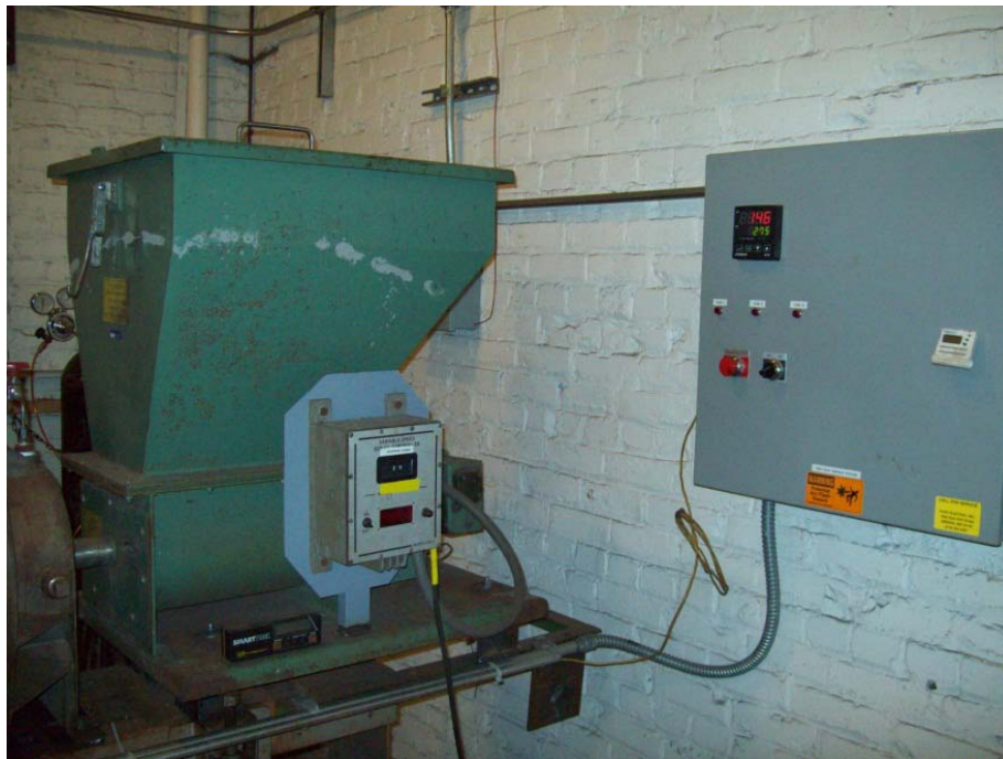
Figure 7: VFD Feeder and Temperature Controller for Calciner Torrefier
