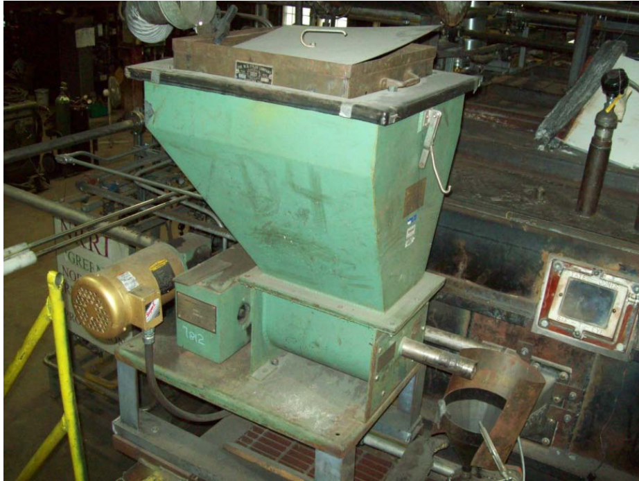
Figure 11: Coal Feeder and Feed Hopper
