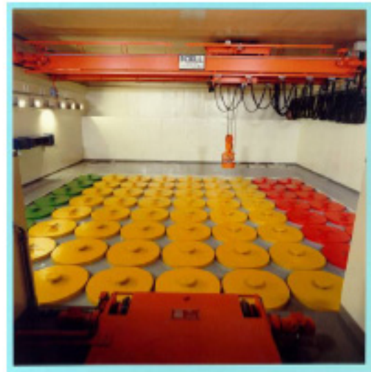
Figure A-5. Spent fuel storage.
