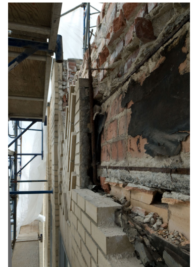
DESTRUCTIVE EXAMINATION (PROBE), UNDERTAKEN DURING THE MASTER PLAN, WHICH REVEALED THE EXTENT OF THE STRUCTURAL PROBLEMS AT THE EXTERIOR ENVELOPE
