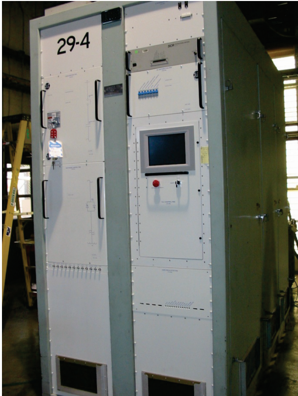
Figure 6. Overall view of the upgraded modulator.
