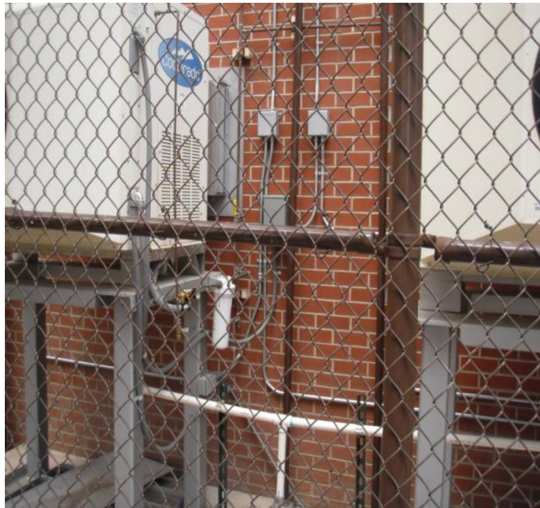
Figure 81. Coolerado drain water piping
