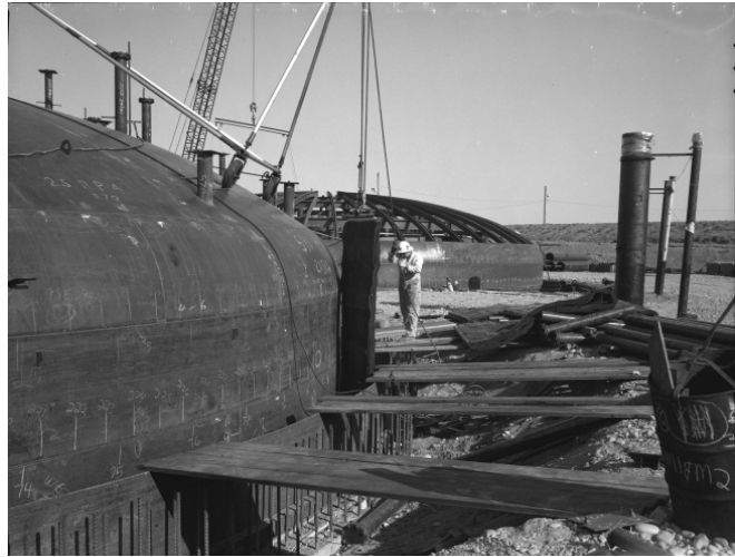
Figure 4-10. Installing Insulation in the Annulus of Tank AY-102 in Preparation of Stress Relieving (Photo No. 50618-3) (Taken 9/12/1969)
