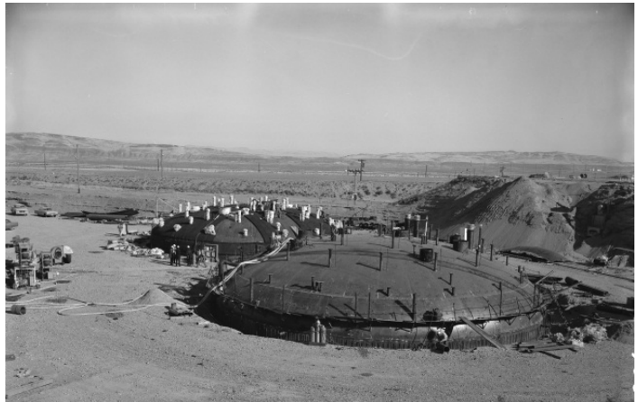
Figure 4-12. Water is Pumped Out of Tank AY-102 (foreground) After Hydrostatic Test While Crews Are Preparing Tank AY-101 for Stress Relieving (Photo No. 50906-13) (Taken 10/24/1969)
