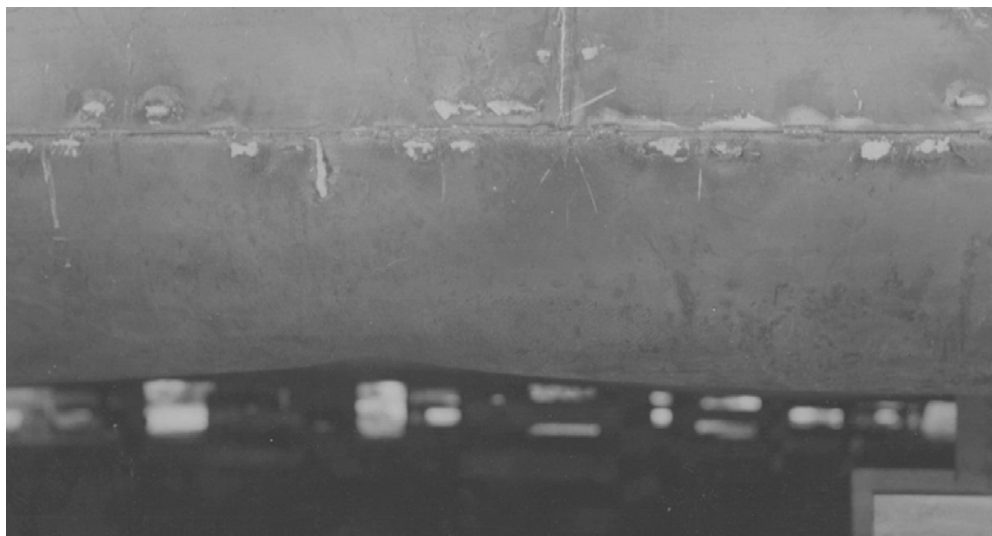
Figure 5-10. Example of Warped Secondary Liner Bottom Knuckle (Photo – 8074)
