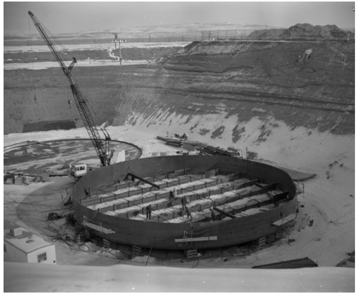
Figure 4-4. Beam Supports in Tank AY-102 for Raising and Lowering the Tank Bottom
