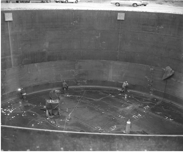
Figure 4-8. Tank AY-101 Completed Primary Bottom and Welding of the First Course Primary Wall (Photo No. 8179) (Taken 6/23/69)
