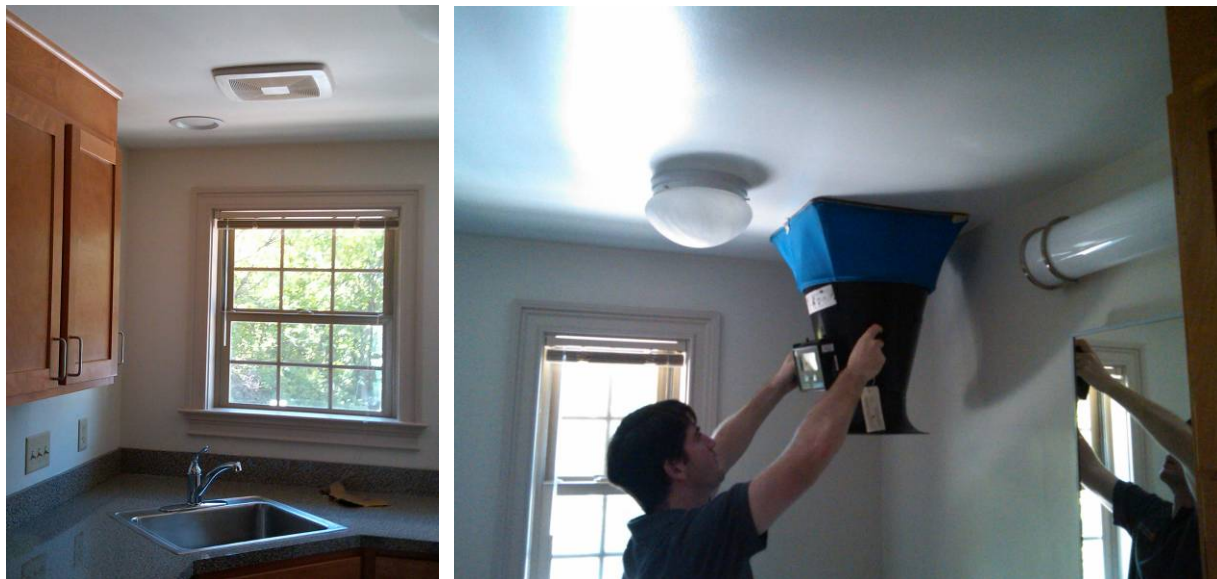
Figure 17. Kitchen room fans and testing bath fan performance
