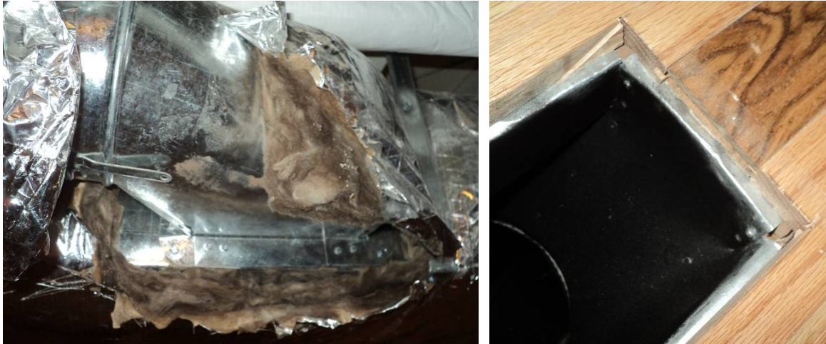
Figure 21. Basement ducts were unsealed in initial units
