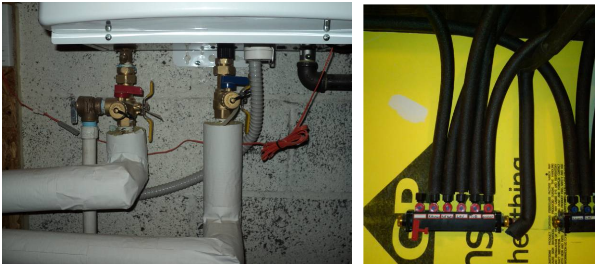
Figure 16. Insulated copper at tankless unit and insulated PEX at branch runs
