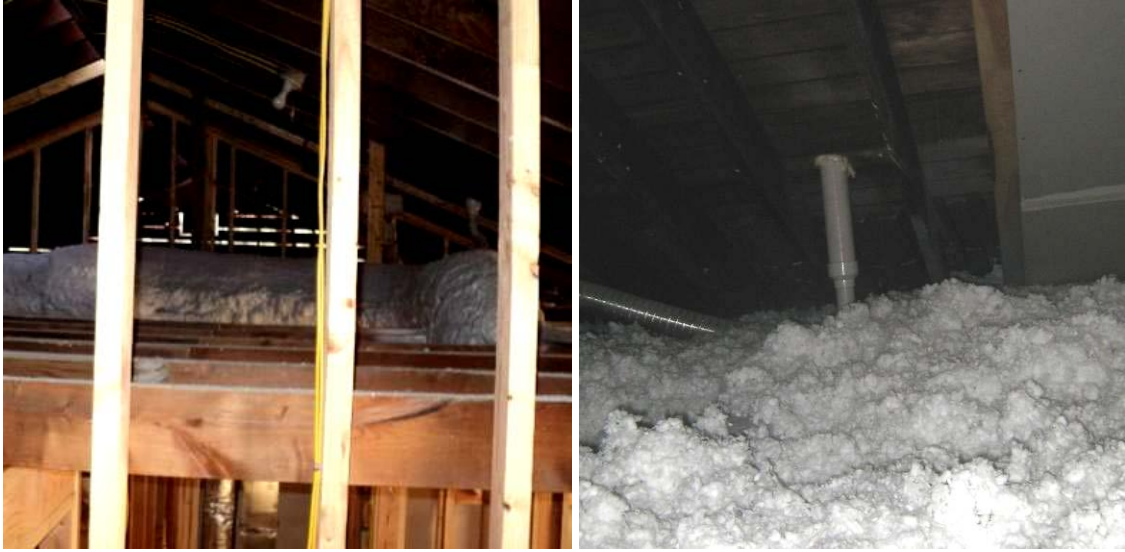
Figure 15. Attic ducts sprayed with ccSPF and buried in blown fiberglass
