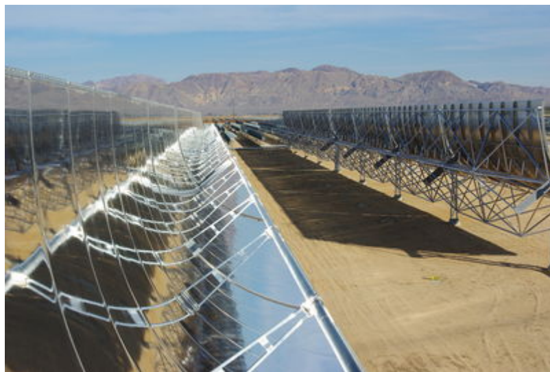
Figure 5-9. Parabolic Trough Undergoing Testing in Southern California
