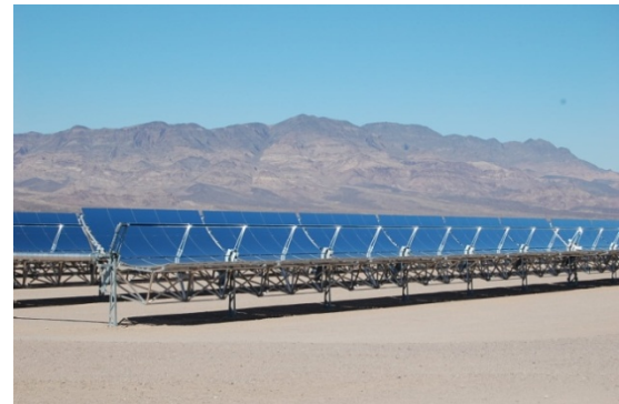
Figure 5-1. Example of a Parabolic Trough Plant
