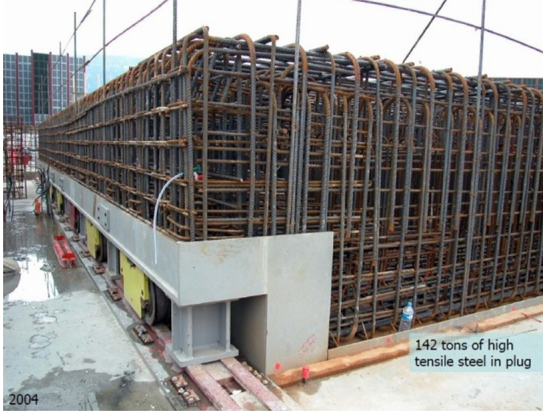
Fig. 11.7: Steelwork of the CMS plug
