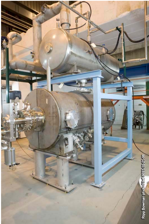
Figure 3. The cryomodule and liquid helium ballast tank installed in the ERL blockhouse.
